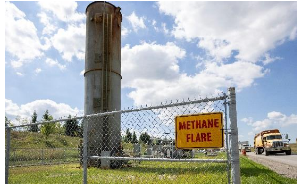
The methane flare stack at the W12A Landfill
