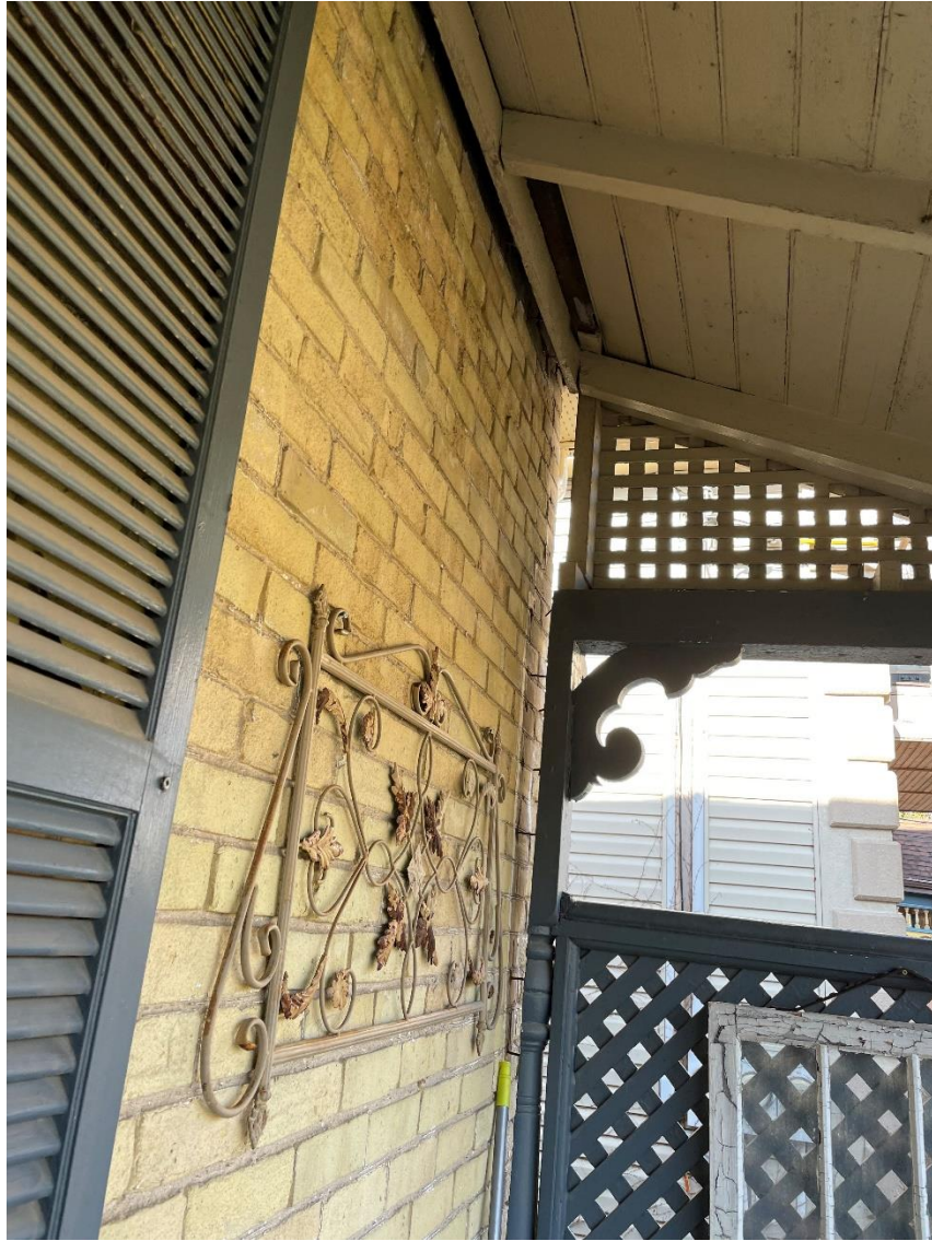
Image 3: Photograph submitted with the Heritage Alteration Permit application demonstrating the need for repairs to the porch at 27 Bruce Street. This photograph also documents the turned posts and bracket detail of the former porch.
