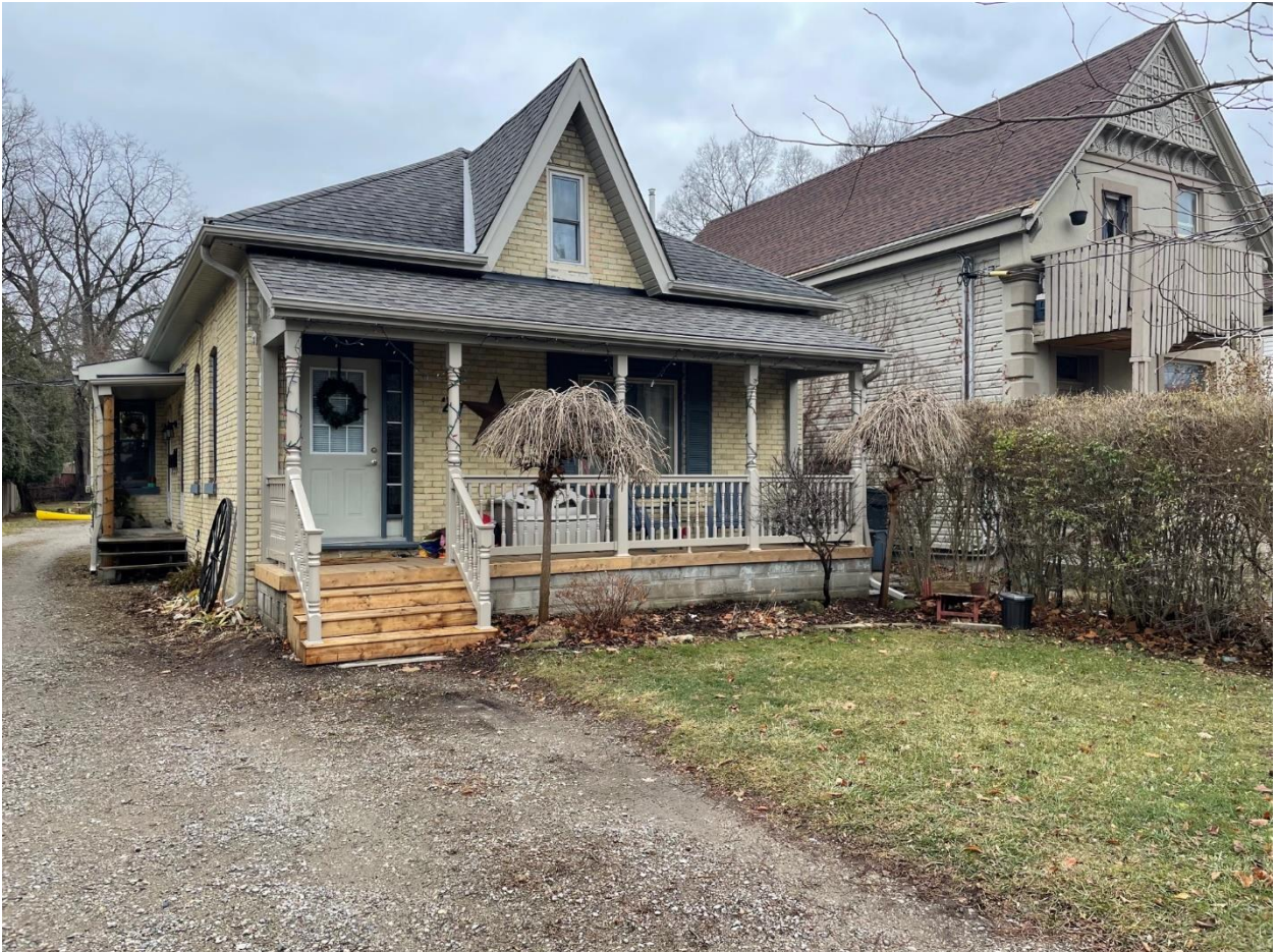
Image 2: Photograph submitted with the Heritage Alteration Permit application showing the porch with vinyl-clad (plastic) posts and vinyl railings, with pressure-treated decking.
