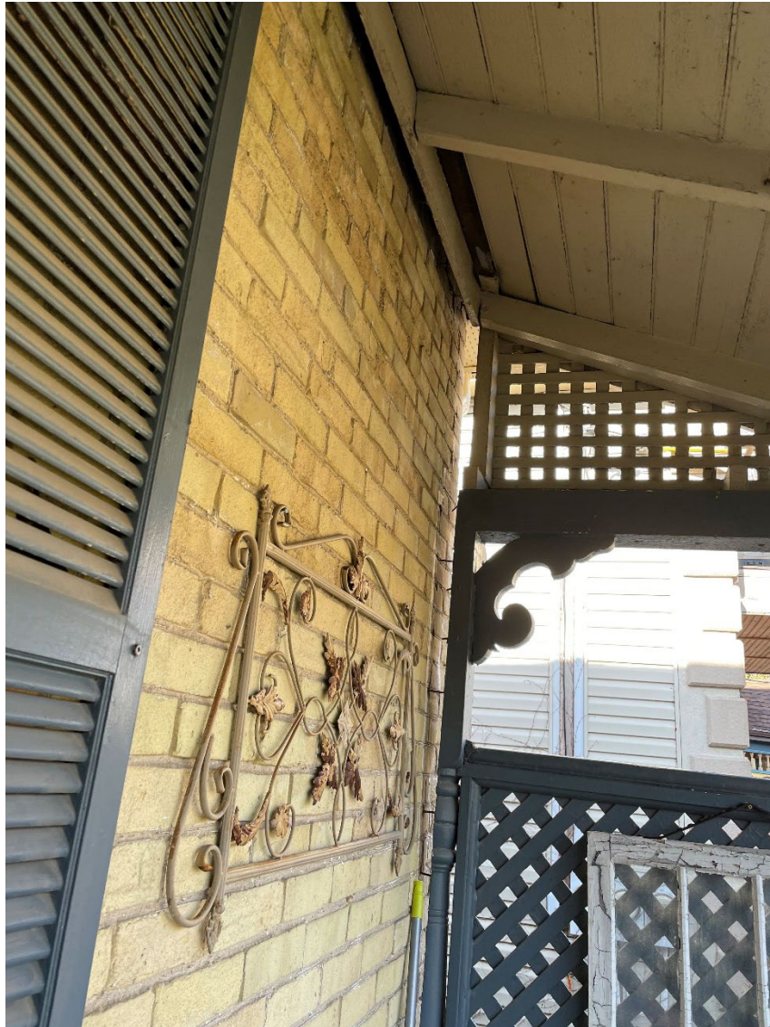
Image 3: Photograph submitted with the Heritage Alteration Permit application demonstrating the need for repairs to the porch at 27 Bruce Street. This photograph also documents the turned posts and bracket detail of the former porch.
