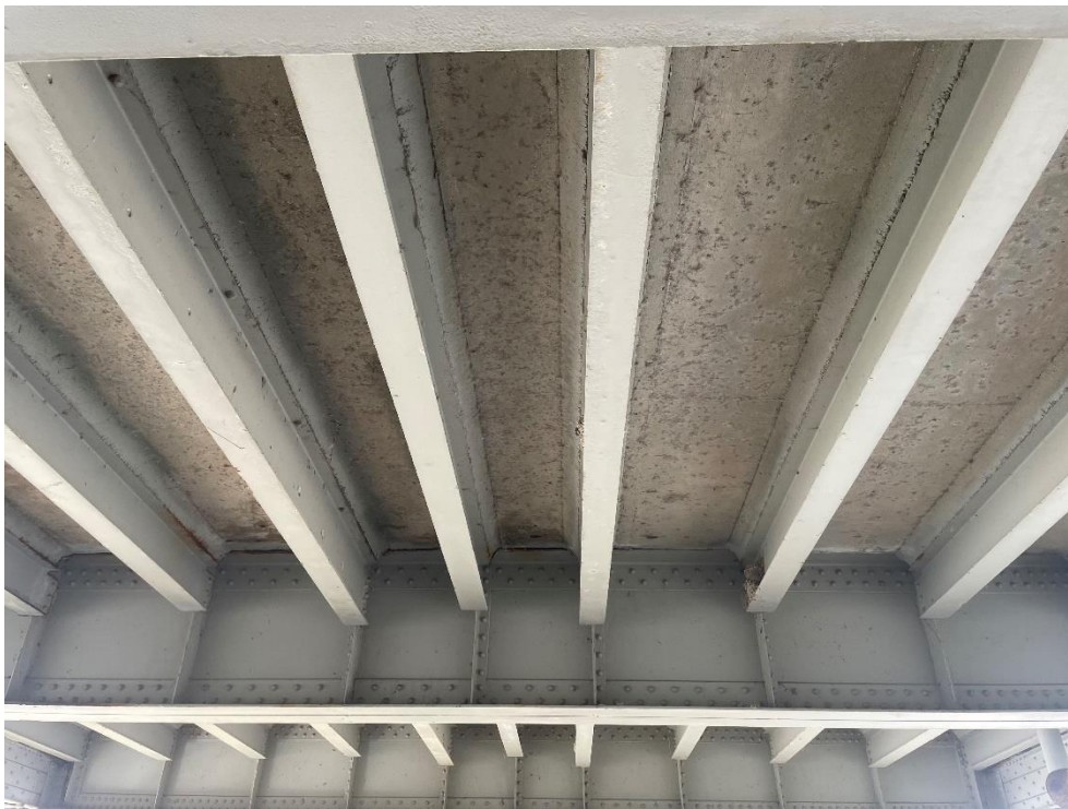
Photograph 25: View of the concrete deck soffit, the steel stringers and steel floor beams (AECOM, April 2023)
