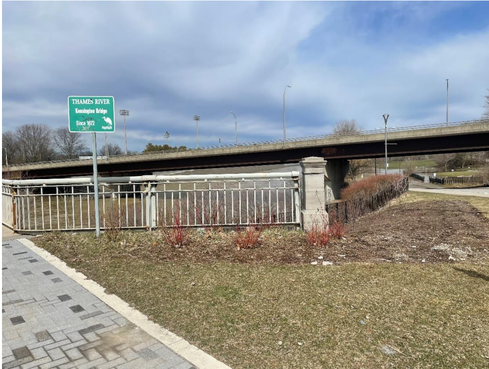
Photograph 18: Northeast original concrete end post connected to the handrailing and Bridge sign: “Thames River, Kensington Bridge, Since 1872” (AECOM, April 2023)
