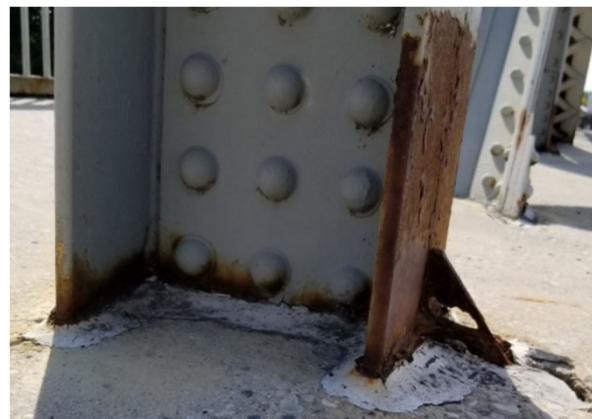
Localized corrosion on bridge truss
