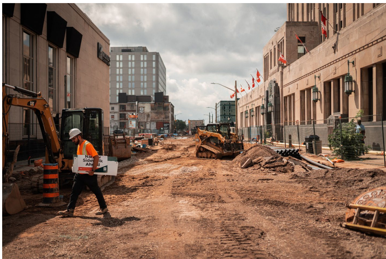
Above: Downtown Loop Phase 2 construction site at Queens Avenue between Richmond Street and Talbot Street.
