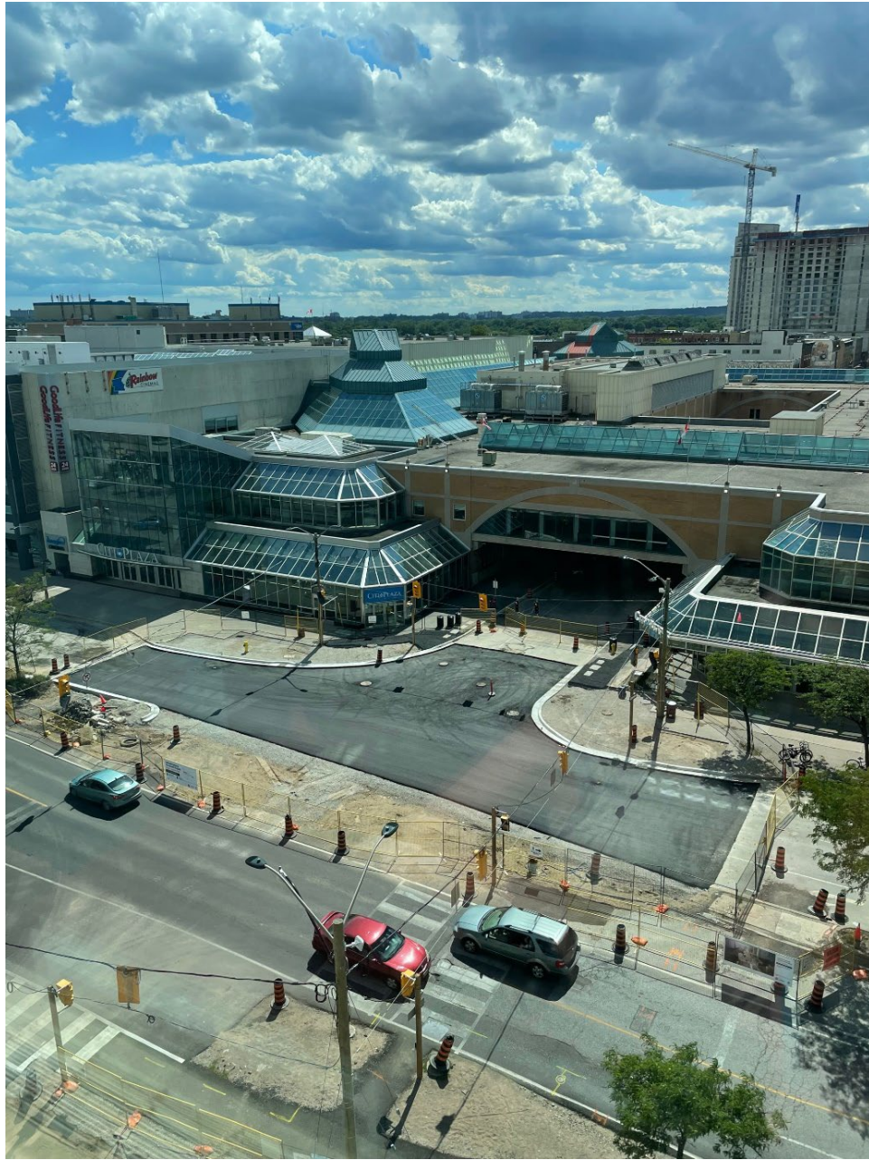
Above: Aerial view of the East London Link Phase 1 construction site at the King Street and Wellington Street intersection.
