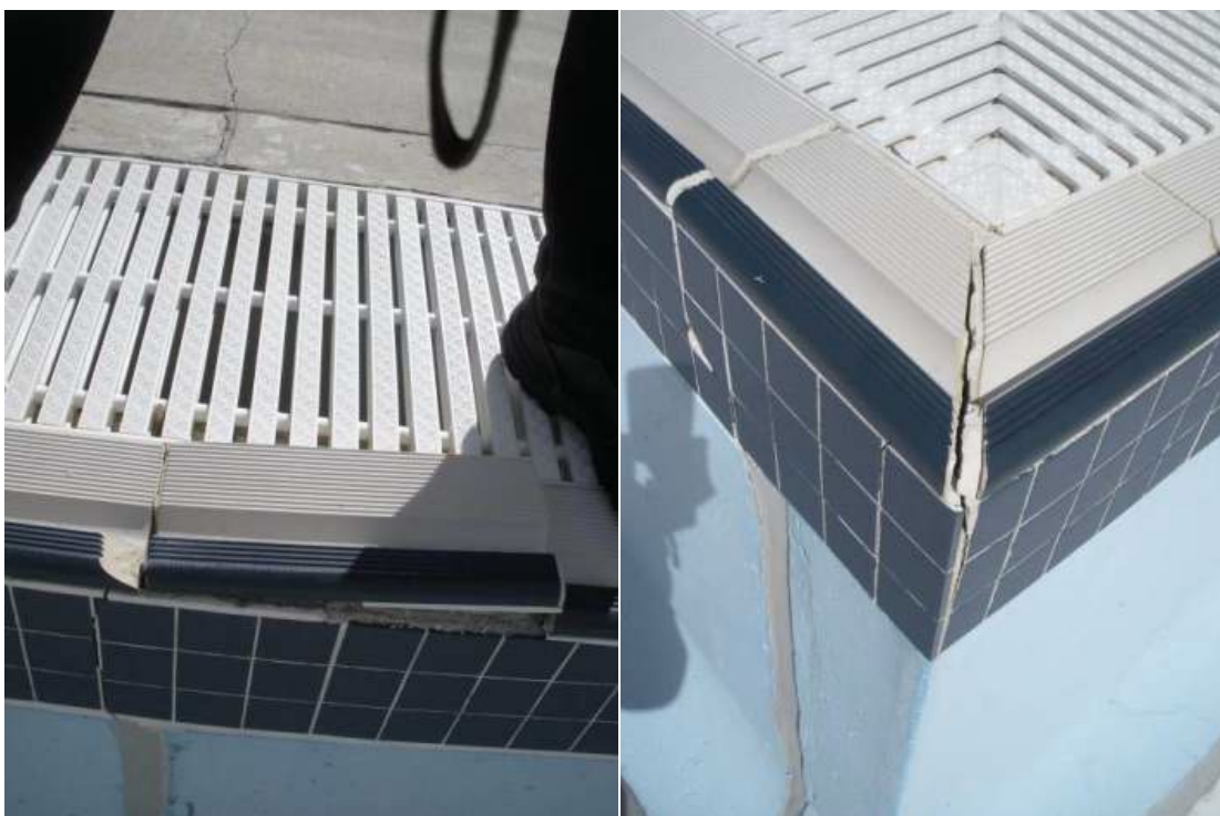
Damage to coping and gutter – indication of pool movement, recently repaired
