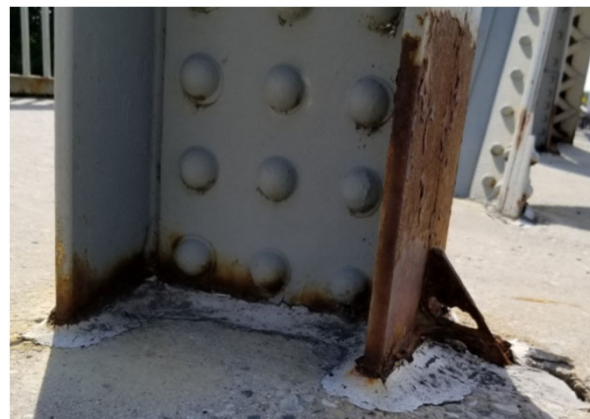
Localized corrosion on bridge truss
