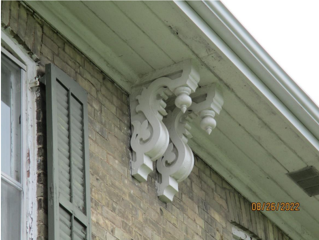
Image 13: Detail showing deep eaves, wood soffit and paired brackets with relief scrollwork and pendant finials, on the Routledge Farmhouse, August 26, 2022.
