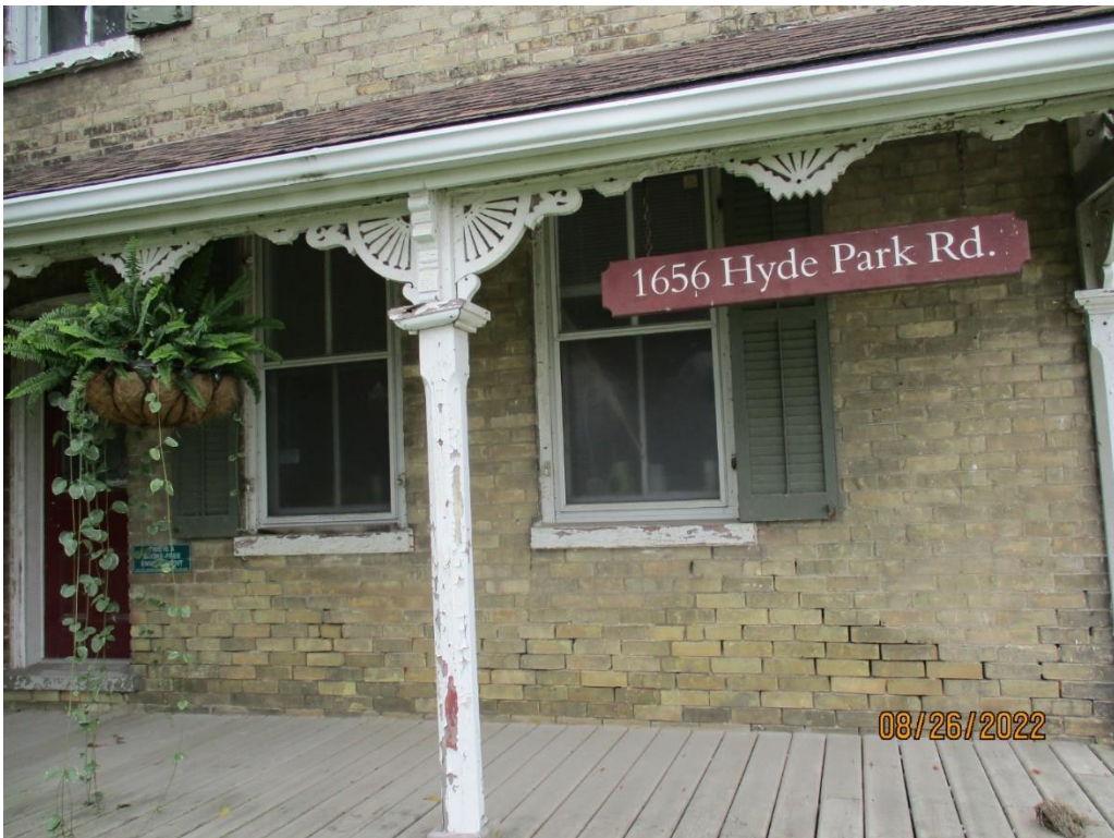
Image 4: View showing the chamfered posts with capitals and fretwork on the existing porch on the Routledge Farmhouse at 1656 Hyde Park Road, August 26, 2022.
