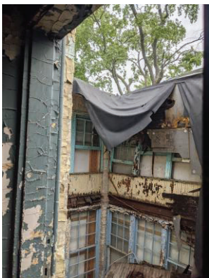
Photo 14: East porch collapse in June 2021
