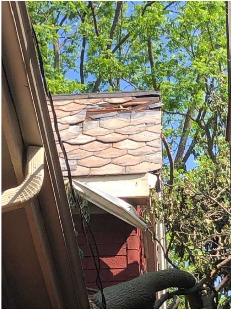
Image 7: Photograph submitted as a part of an inspection report showing extent of damage to the slate roof.
