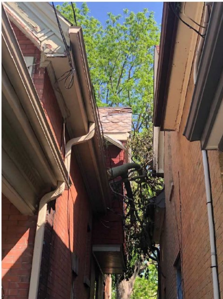
Image 8: Photograph submitted as a part of an inspection report showing extent of damage to the slate roof.
