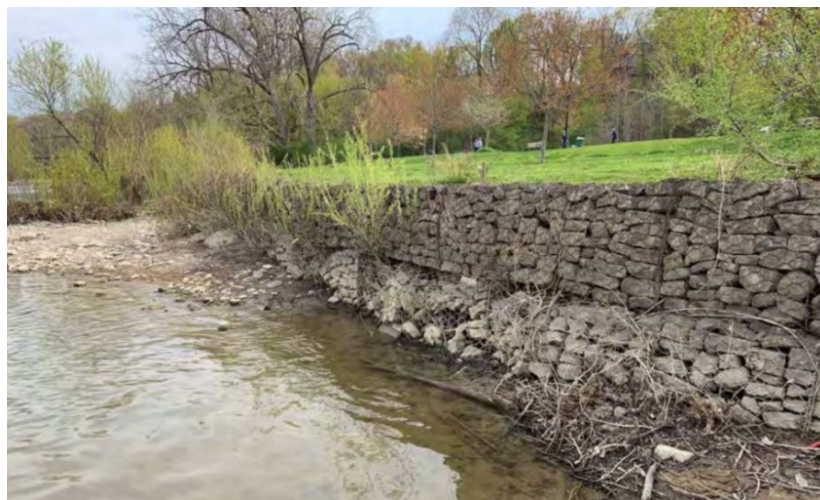
Figure 2: Harris Park, partial failure of gabion retaining wall (2021)
