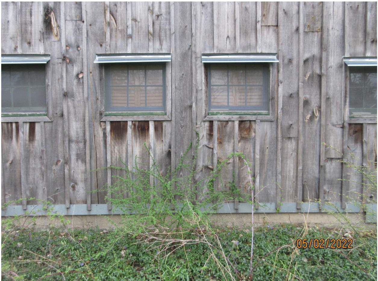
Image 4: Detail of four of the horse stall windows on the east façade of the building at 514 Pall Mall Street. There are fourteen horse stall windows on the building, articulating its origins as a stable.
