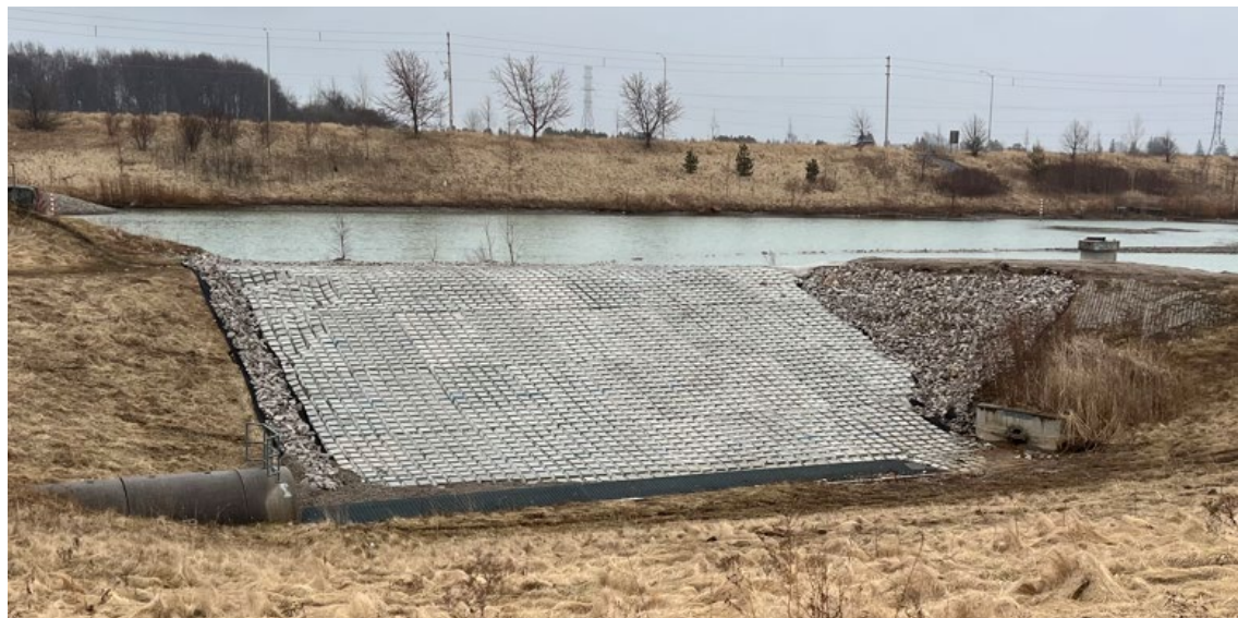
Figure 2: a) Failed turfstone spillway at Summerside SWMF (2020), b) Upgraded cable concrete spillway showing failure along the north section (2022)
