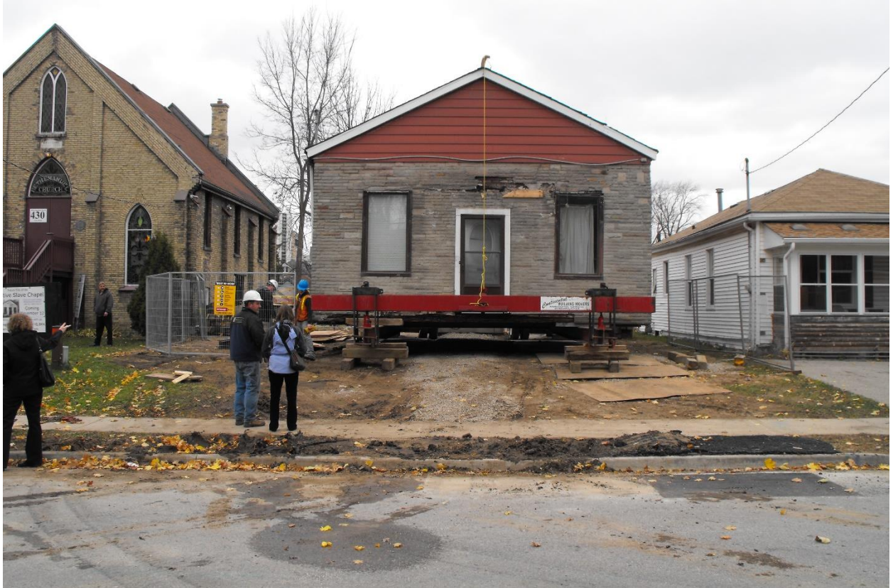
Image 4: The Fugitive Slave Chapel being set into its present location at 432 Grey Street on November 12, 2014.
