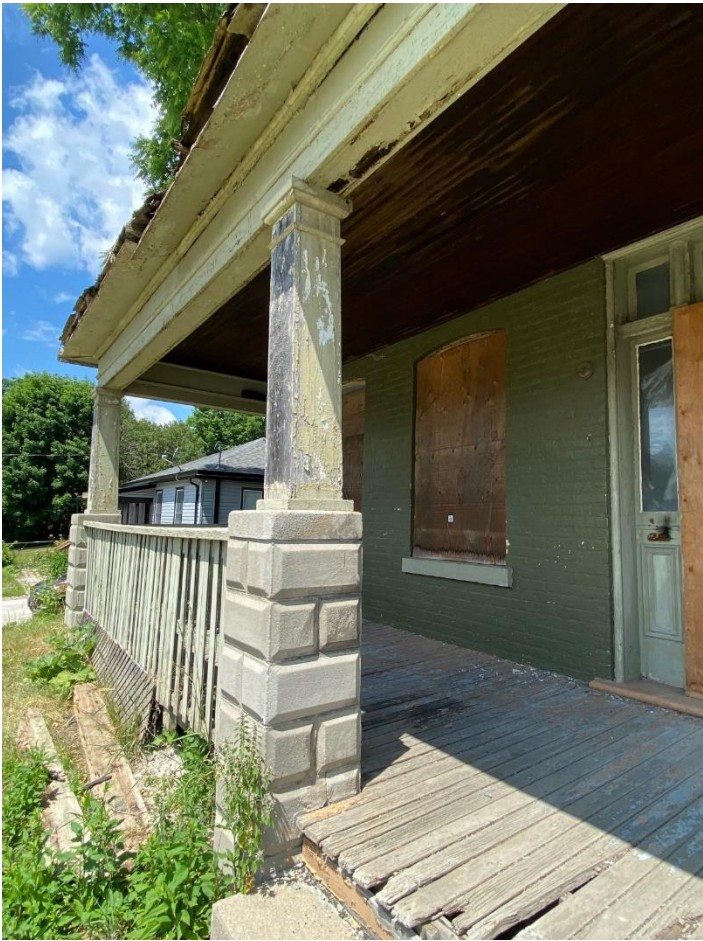
Image 10. Porch supported by concrete blocks and wooden posts
