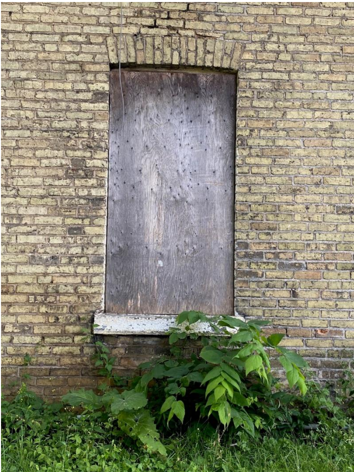
Image 14: Detail of boarded-up window opening – 1 st floor, west elevation – showing shallow arch with voussoirs and two-over-two (2/2) wooden window frame and wood sill
