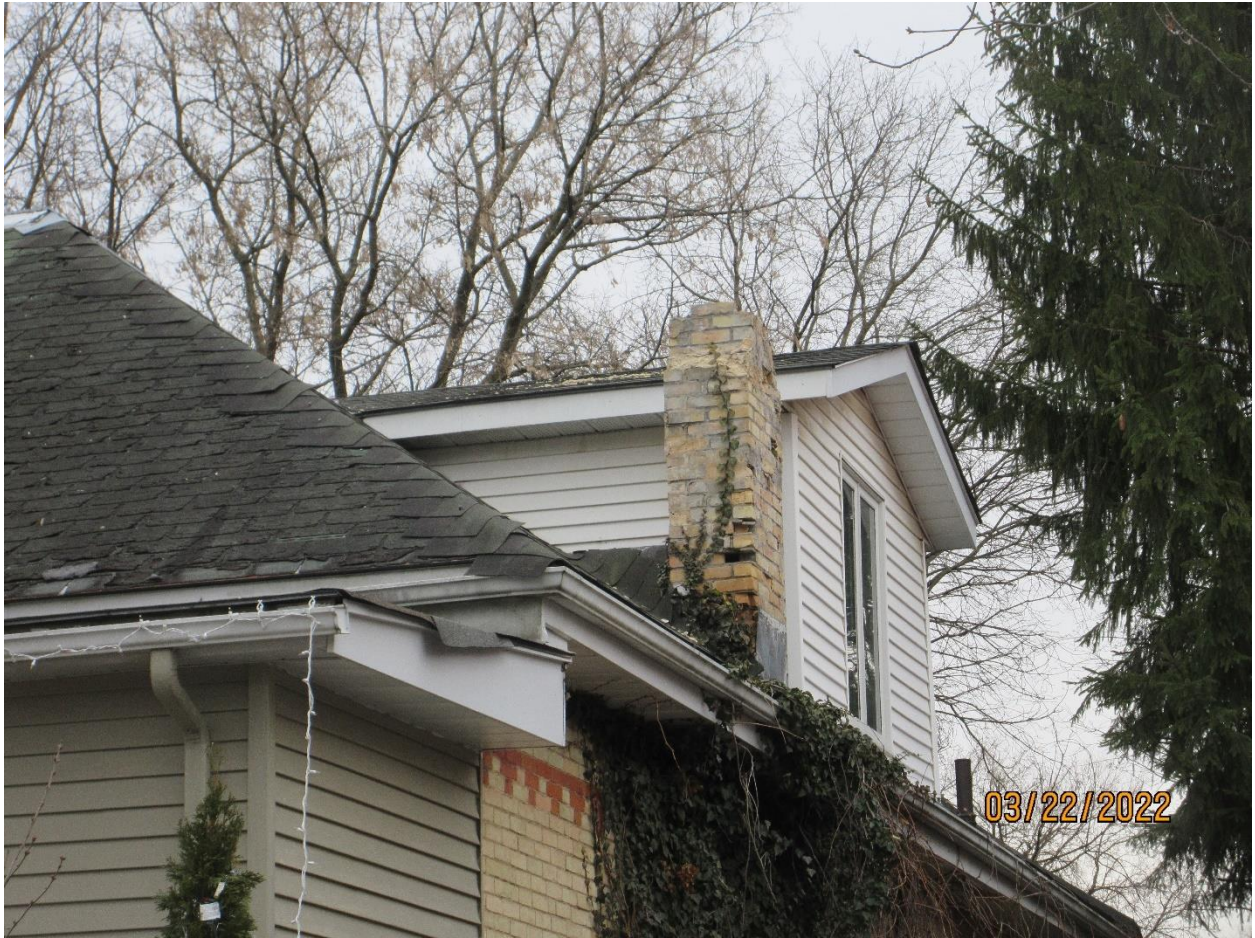
Image 9: Photograph showing the partially collapsed chimney on the subject dwelling at 45 Bruce Street (2022).
