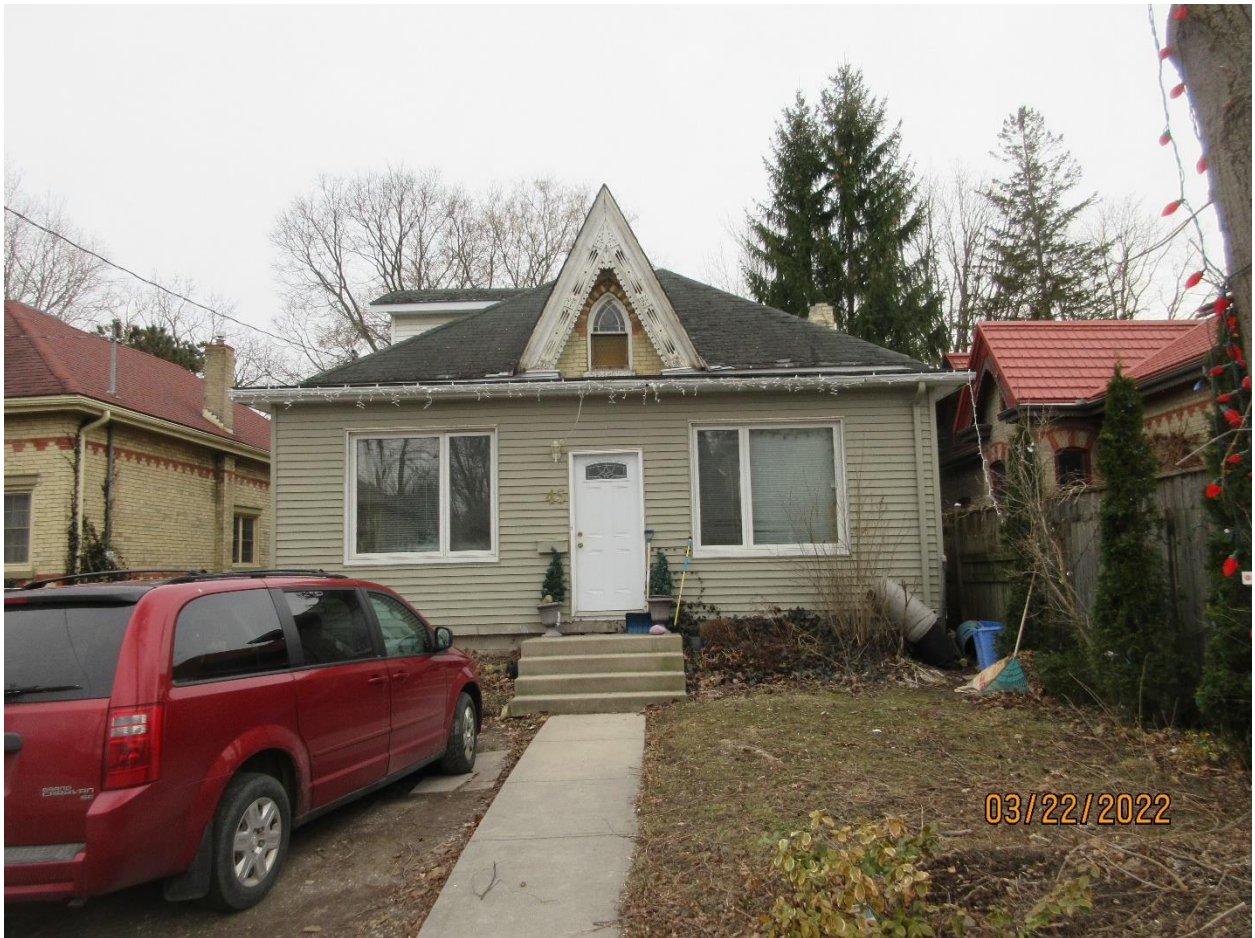
Image 7: Photograph of the subject dwelling at 45 Bruce Street, shortly after the partial collapse of the chimney (2022).
