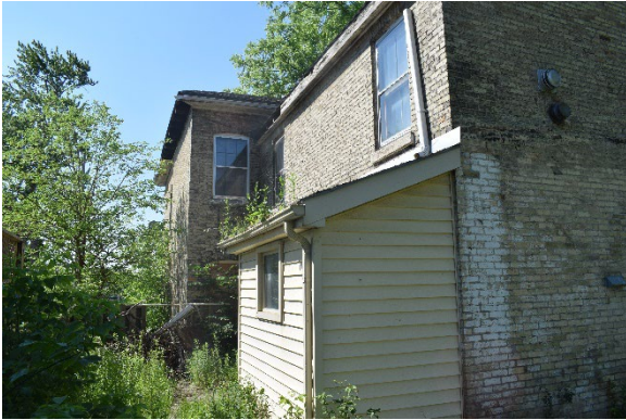
Plate 24: Looking south showing second storey windows and shed roof addition of east elevation
