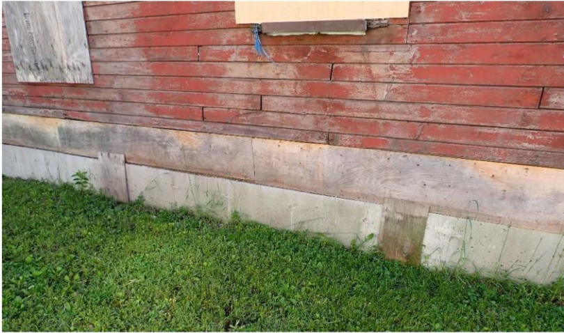
Photographs 3 : Slots in top of foundation wall to install beams for lifting the building.
