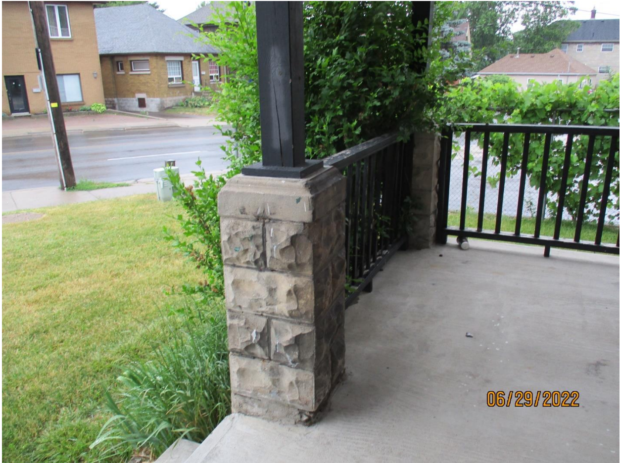
Image 3: Photograph showing porch details on the dwelling at 672 Hamilton Road. Note, the posts and railing system have been replaced.
