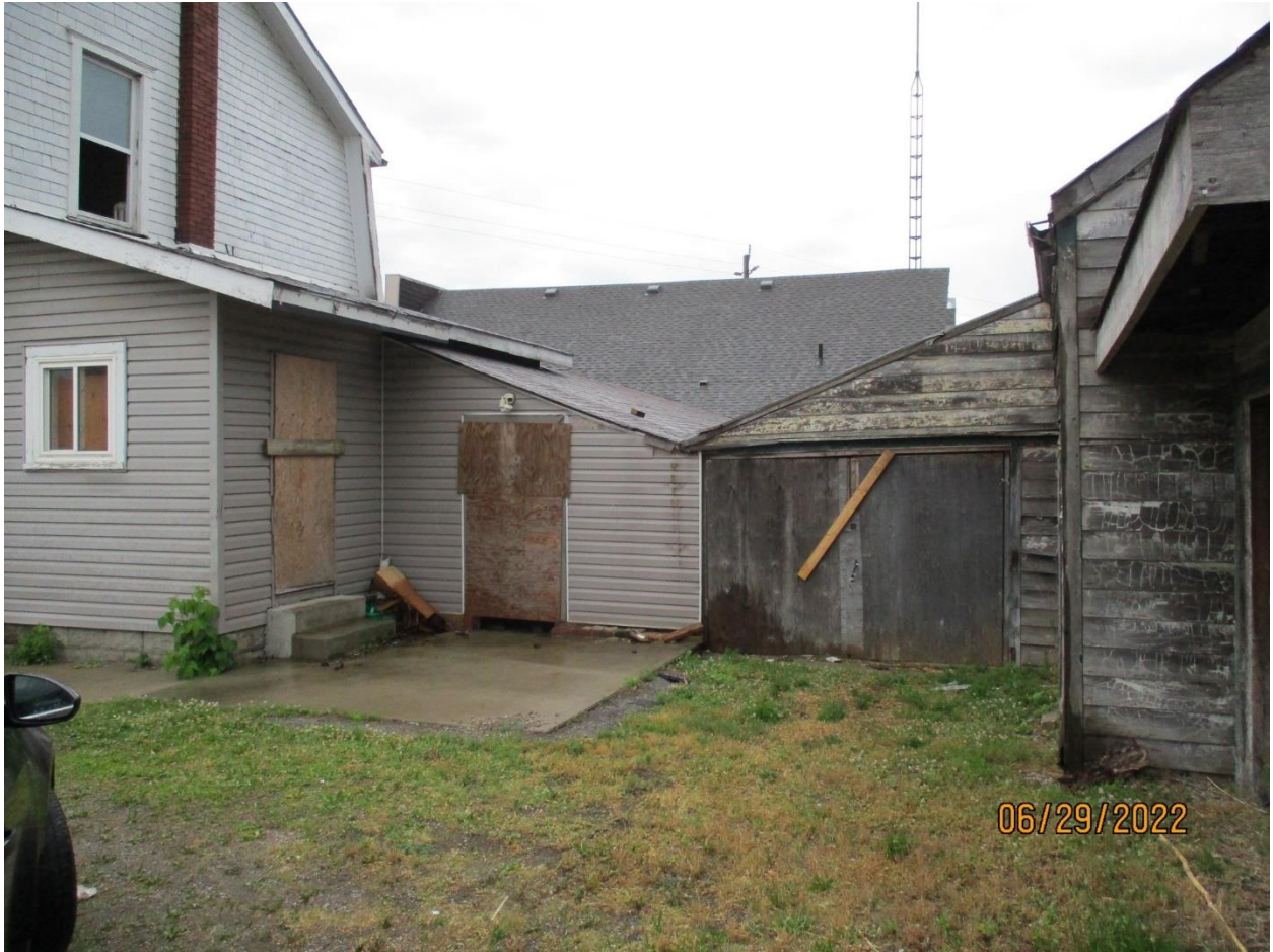
Image 7: Photograph showing the rear additions on the subject property at 672 Hamilton Road.
