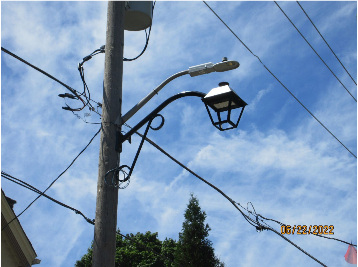
Image 5: Photograph of the new heritage sympathetic light fixture, contrasted to the standard “cobra” light fixtures, being installed on English Street. The “cobra” light fixtures will be removed.
