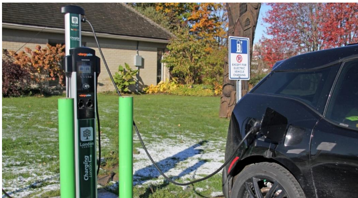
Electric vehicle charger at the Tourism London office on Wellington Street
