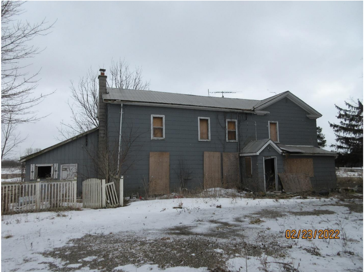
Image 5: View of the north elevation of the farmhouse at 3700 Colonel Talbot Road.
