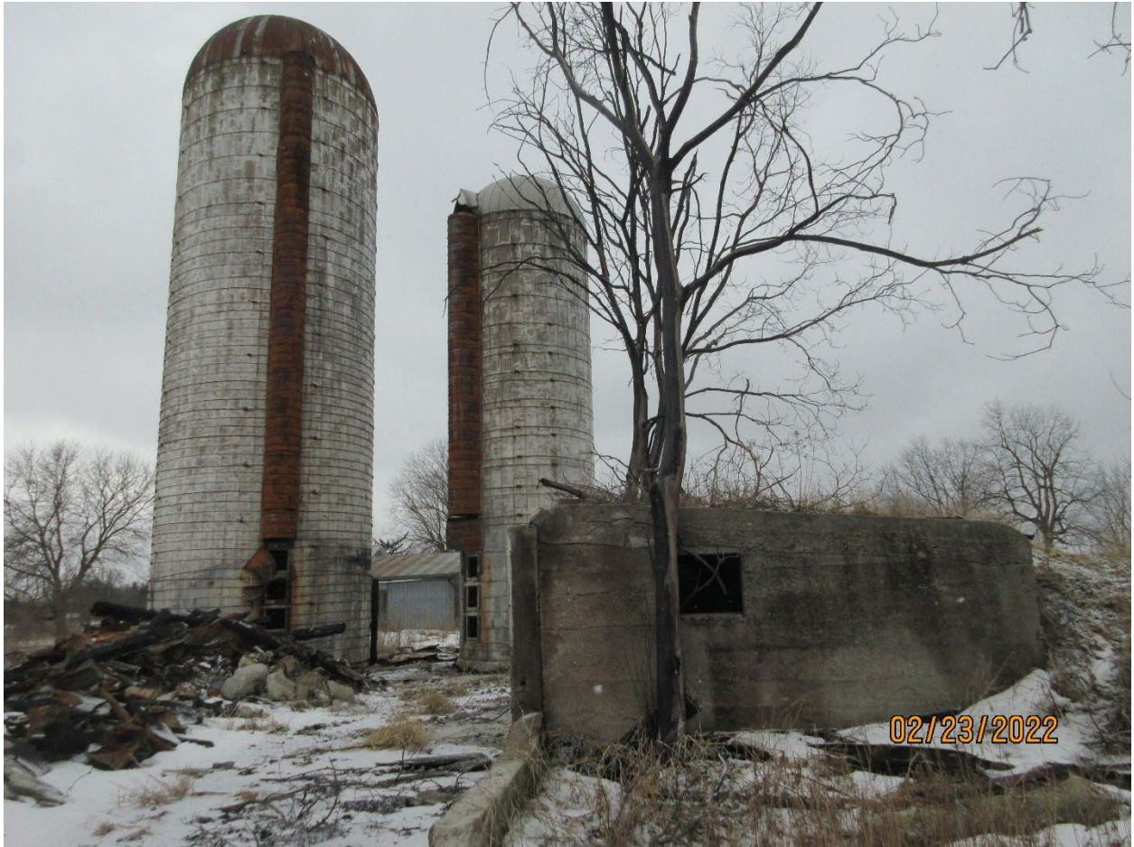
Image 15: View of the silos, showing one of the concrete gangways (barn hill).
