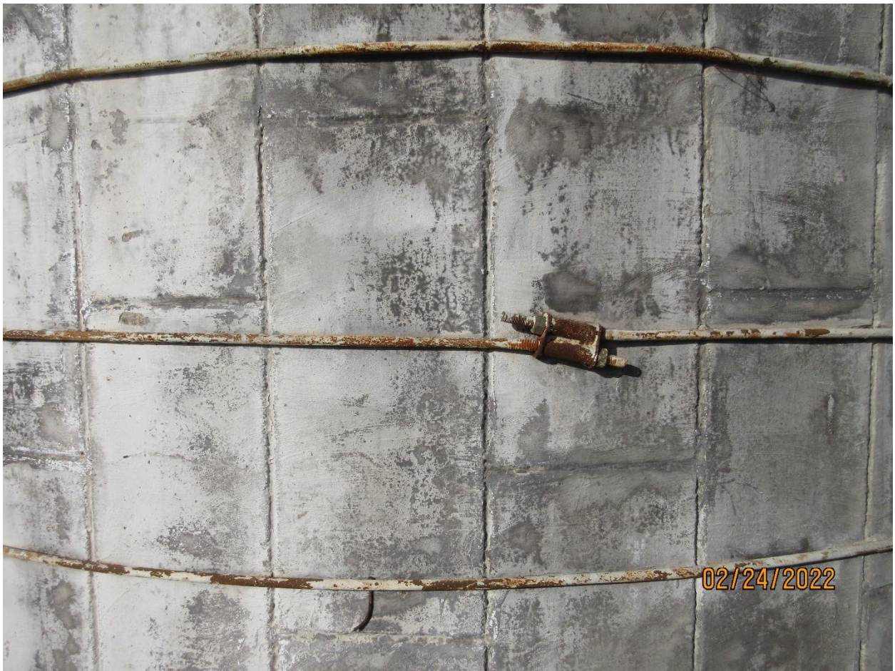
Image 16: Detail of the concrete block masonry, approximately 12" by 30", of the silos with the iron banding.
