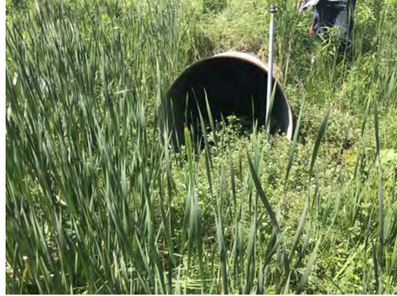
Photo 2 - June 16, 2021 Trib. C, N of Gideon Dr., looking S towards culvert inlet.
