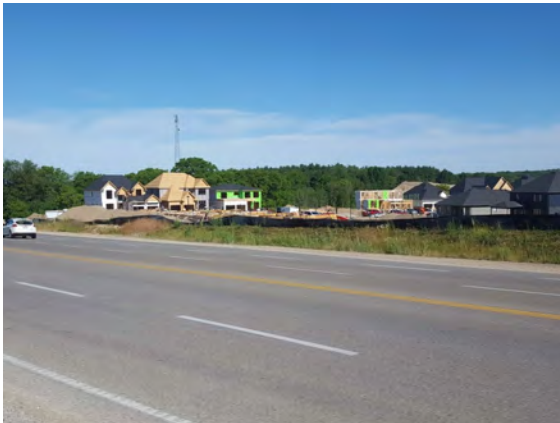
Photo 21 - June 16, 2021 Eagle Ridge Subdivision and right-of-way, looking NW from S side of Oxford Street West.
