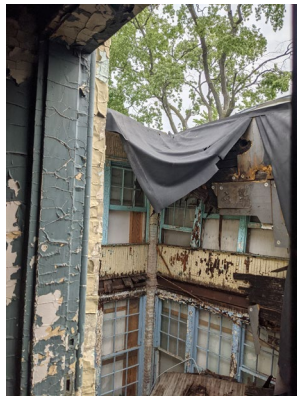
Photo 14: East porch collapse in June 2021
