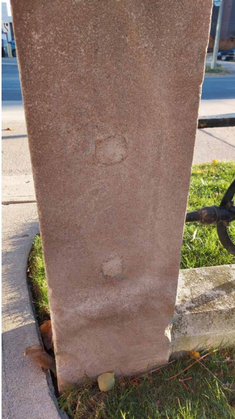
Photograph 20: Former holes in the end posts (for horizontal rail attachment) that were patched up, potentially indicating the end post was turned for repairs (AECOM, November 2021)
