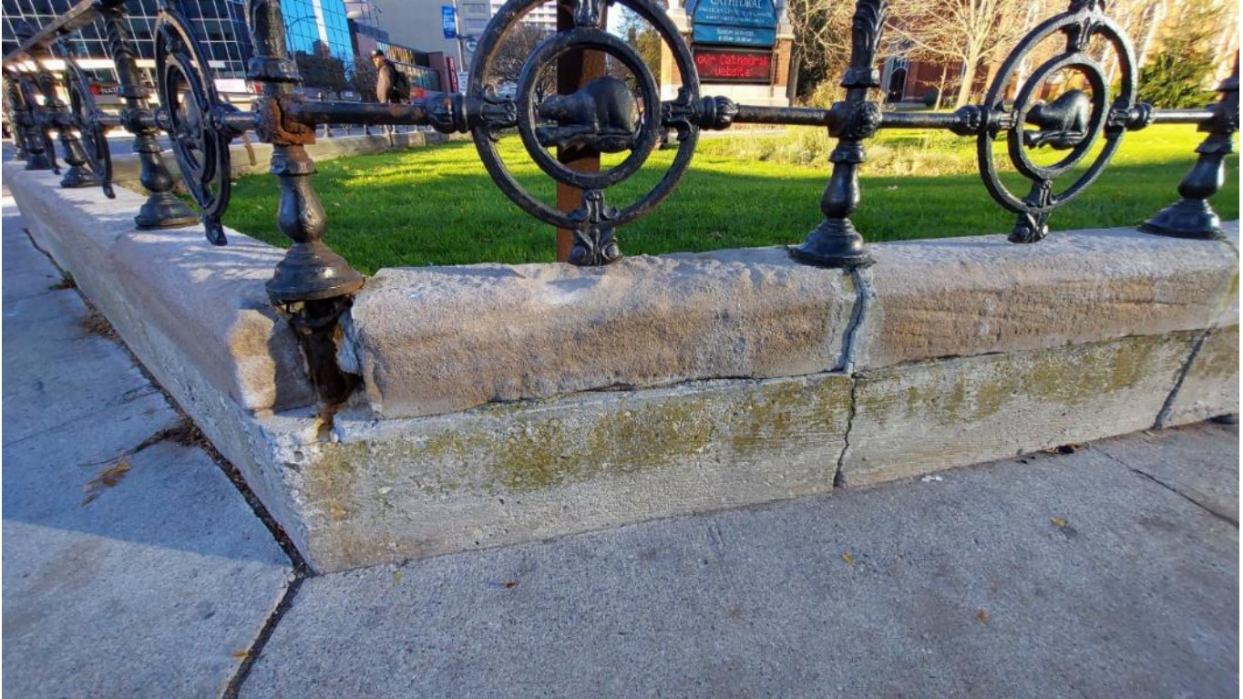
Photograph 22: Example of a cap stone in poor condition (AECOM, November 2021)
