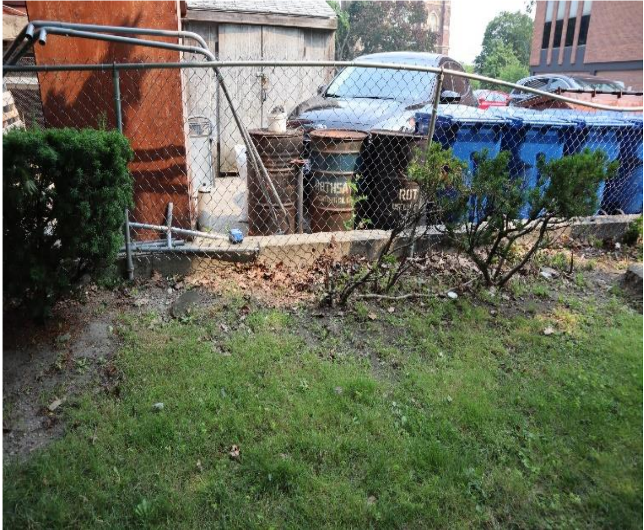
Photograph 5: Northern boundary of the property, showing the foundation of the former fence (AECOM, July 2021)
