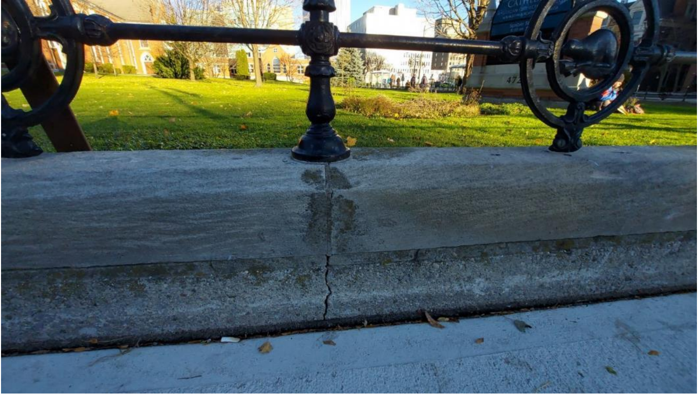
Photograph 27: Caulking below the base of the post to increase contact and seal area below (AECOM, November 2021)
