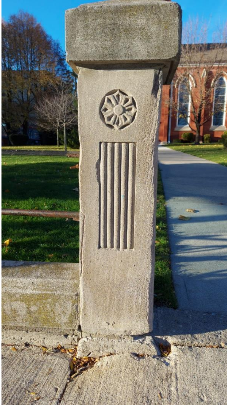
Photograph 15: End post proposed for relocation on Queens Avenue, showing signs of weathering and localized weathering on corners (AECOM, November 2021)
