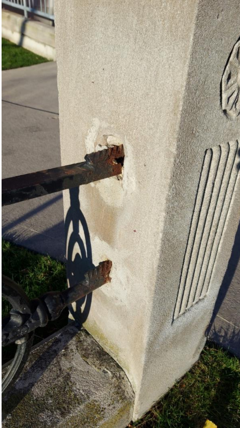
Photograph 18: Original arrangement with where horizontal rails mortared into end posts (AECOM, November 2021)
