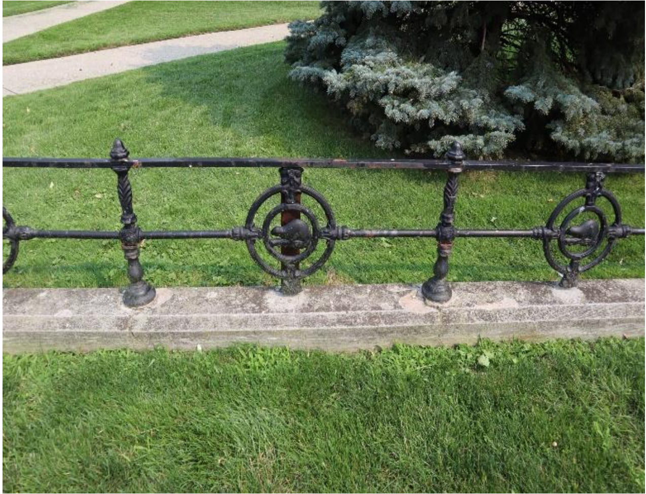
Photograph 35: View of the beaver fence on Queens Avenue with buried foundation (AECOM, May 2021)
