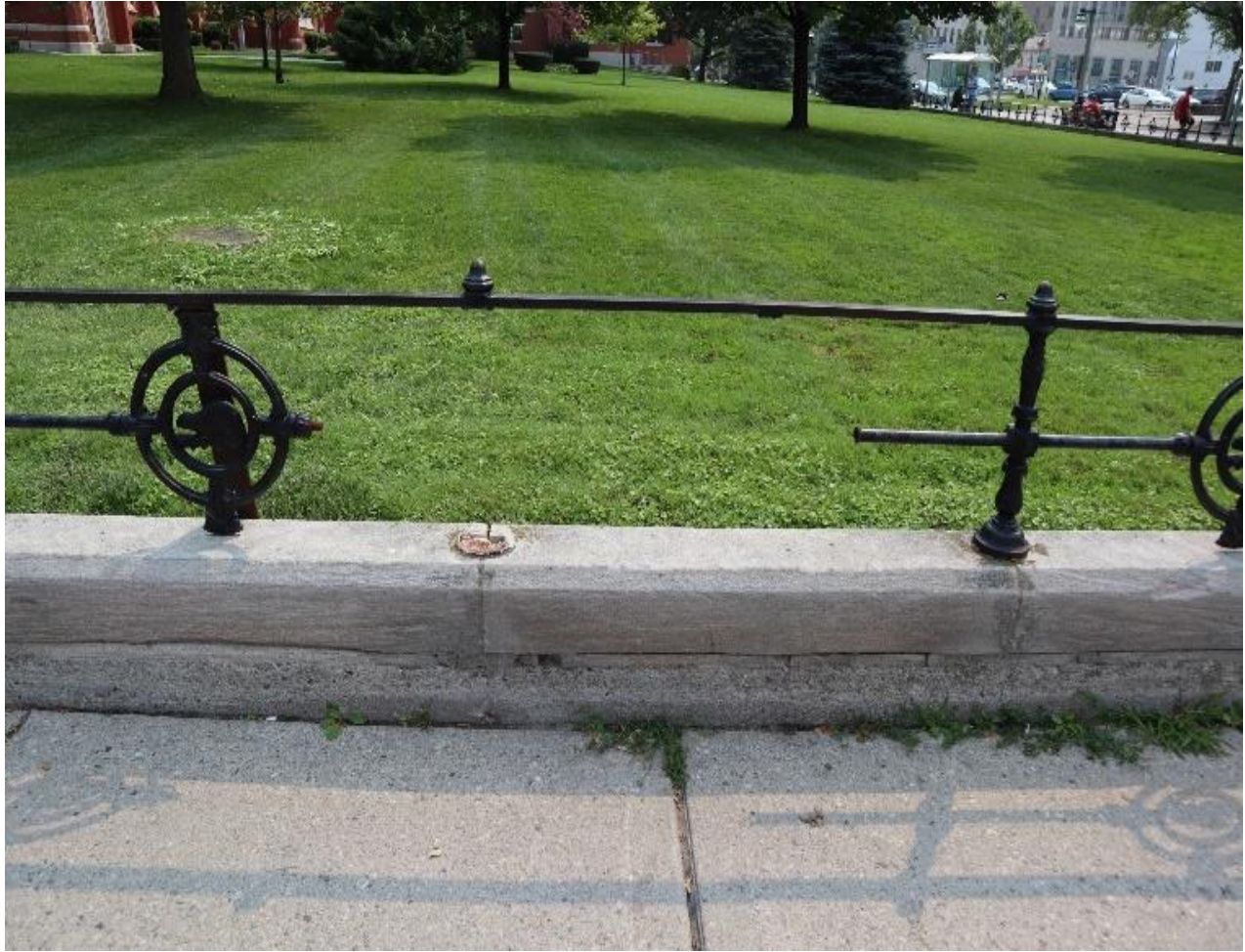
Photograph 26: Missing section of the beaver fence on Richmond Street (AECOM, May 2021)
