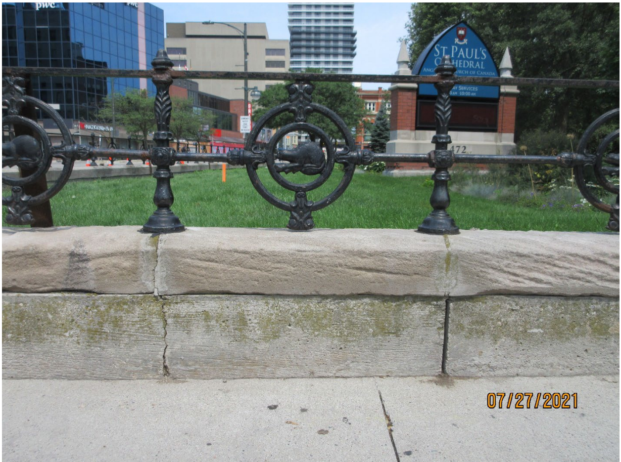
Image 4: Detail view of a typical panel of the beaver fence, composed of its cast iron posts, rails, and medallions, sandstone cap stones, and concrete foundation.
