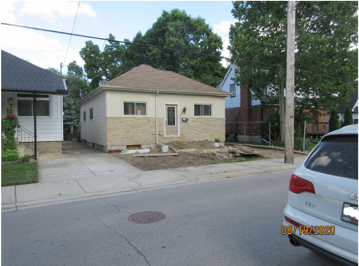
Image 1: Photograph of the dwelling located at 59 Albion Street in August 2020, showing foundation repair work being undertaken, necessitating a restored front porch.
