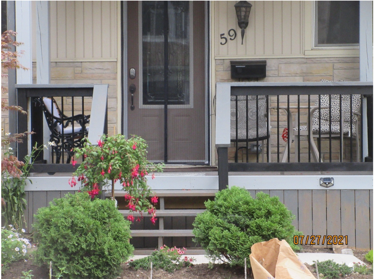
Image 5: Detail of the railing system on the property at 59 Albion Street showing the unapproved NUVO Iron railing system, July 2021.
