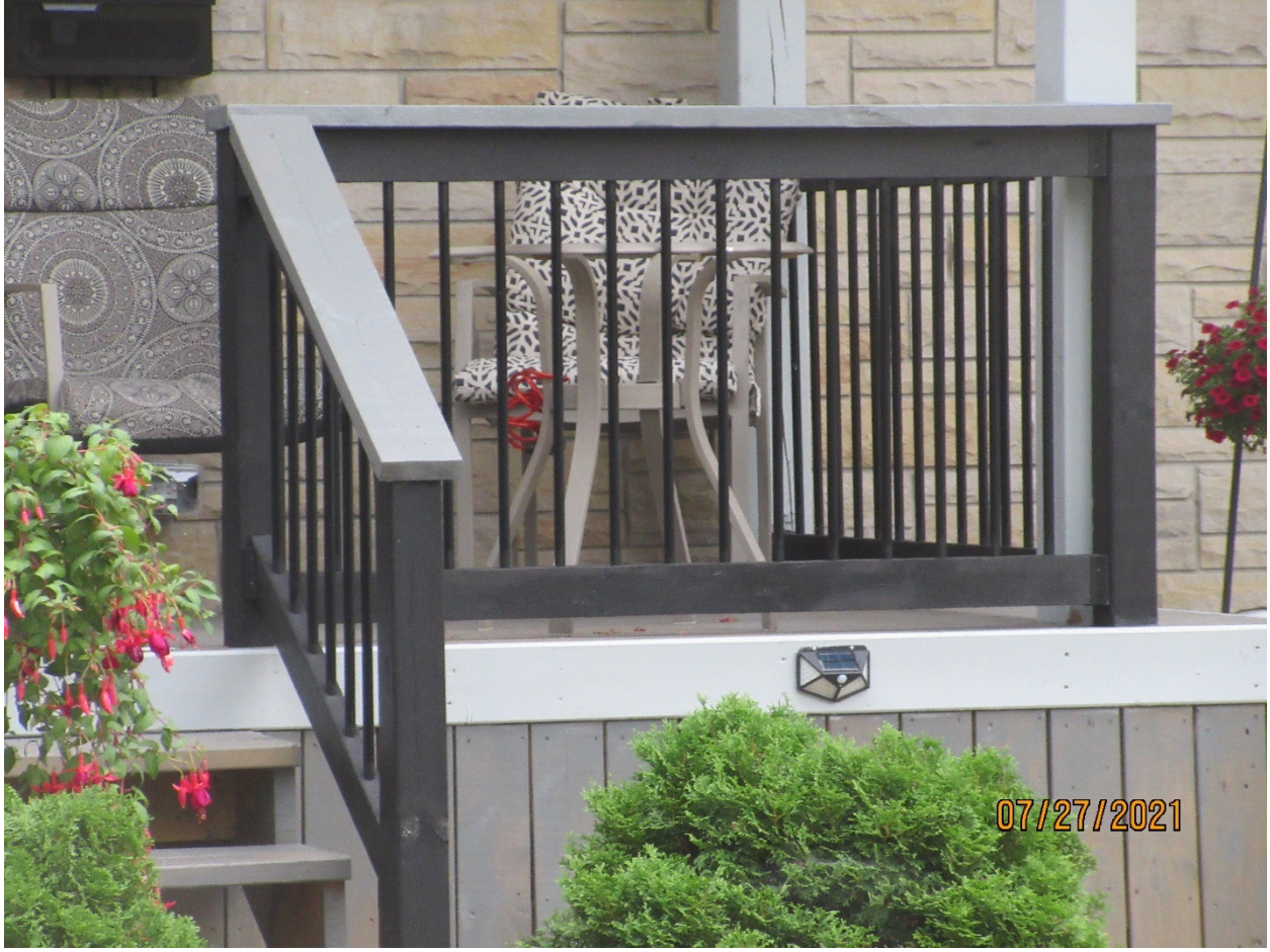
Image 6: Detail of the railing system on the property at 59 Albion Street showing the unapproved NUVO Iron railing system, July 2021.
