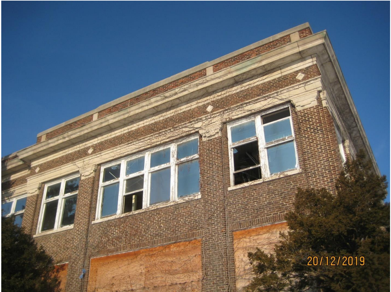
Image 5 Photograph showing pilasters, cornice, and tapestry brick detailing on the Health Services Building.
