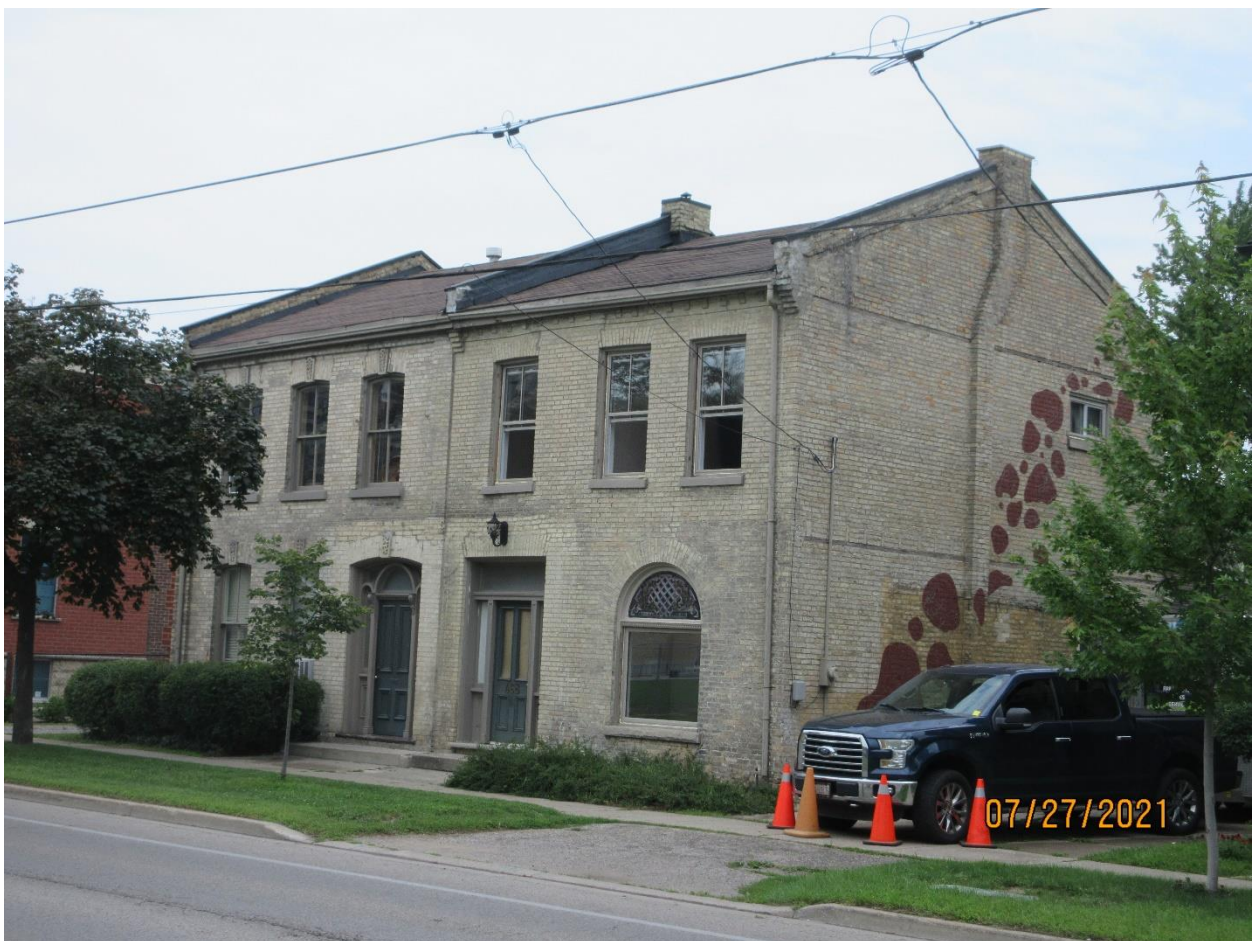
Image 4: Photograph showing the unapproved alterations to the windows at 468 Queens Avenue underway, July 2021.
