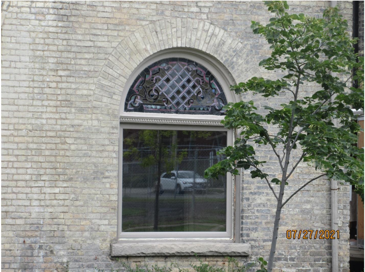
Image 5: Photograph showing the unapproved alterations to the windows at 468 Queens Avenue underway, July 2021.
