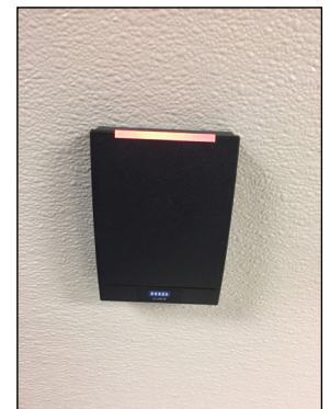
Example of proximity card reader system with visual indicator, City of London.
