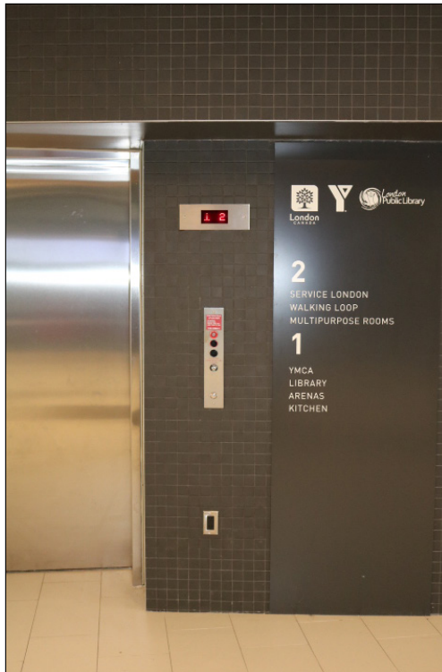
View of an accessible elevator and typical features in lobby, City of London
