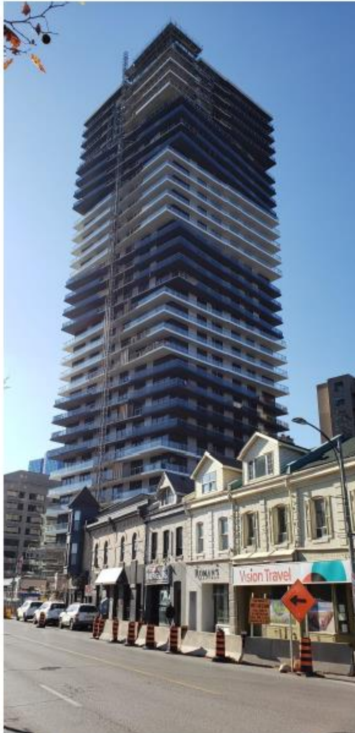
517 Richmond Street a 31-story building nearing construction completion November 14, 2020. This residential building is across the street from the Victoria Park Secondary Plan and it overlooks Victoria Park.
