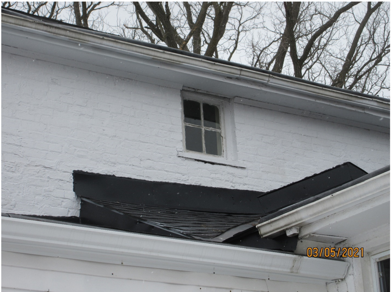
Image 8: The small, four-pane window on the north elevation, under the eaves, in the second storey of the Clarke House.
