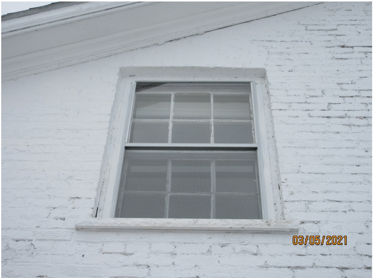
Image 16: Detail of the upper south window on the east elevation of the Clarke House. The sill was previously replaced.
