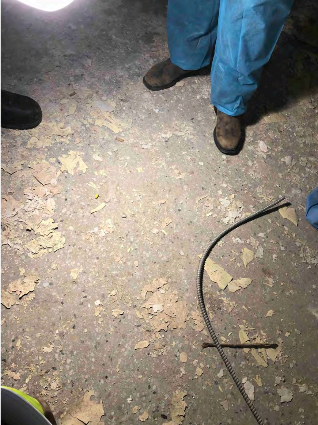
MAIN FLOOR – TERRAZZO FLOORING – the floor is littered with dust and debris but the terrazzo appears to be in fair to good condition
