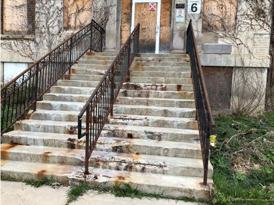
MAIN ELEVATION – STEPS TO THE FRONT ENTRANCE – concrete stairs are severely deteriorated
