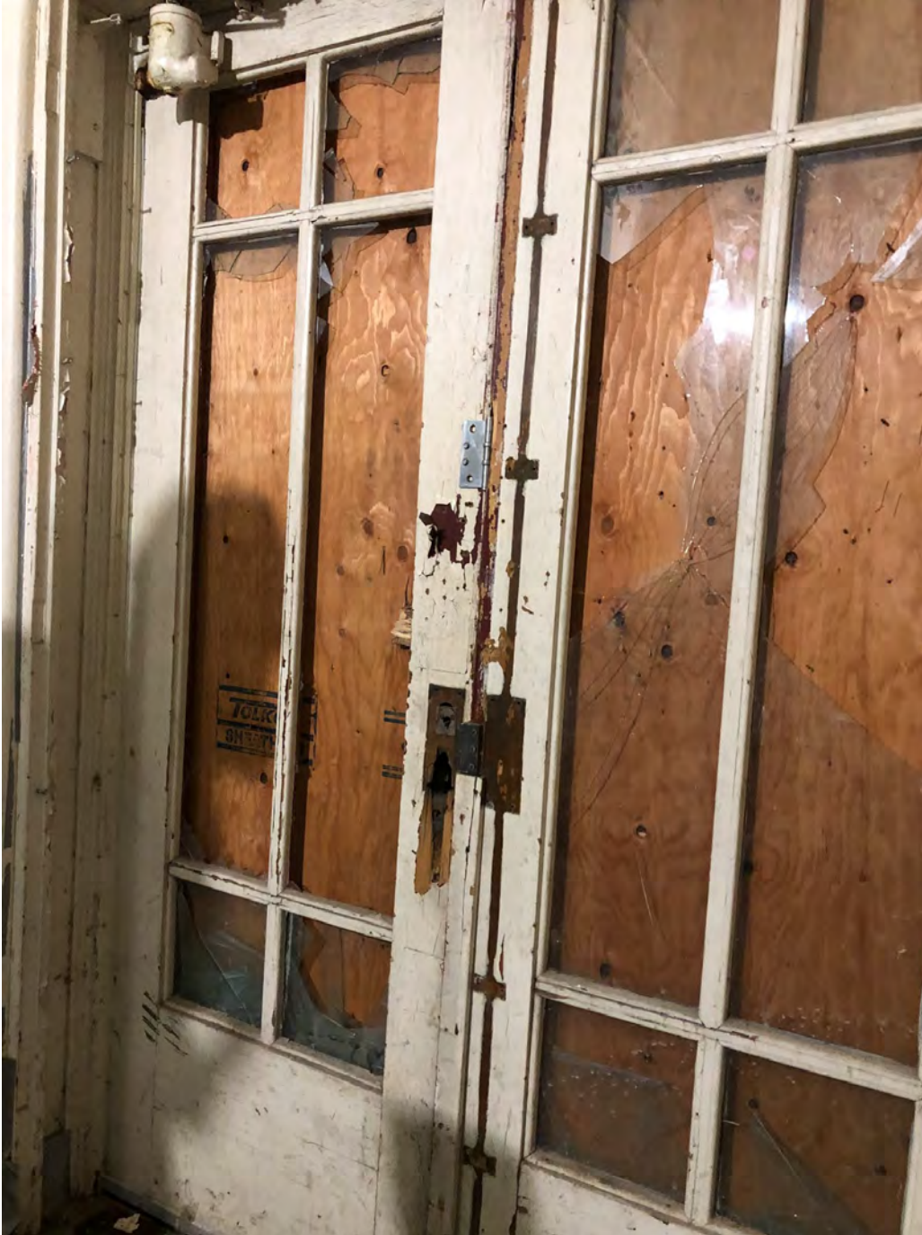
WOOD DOORS – wood doors at the main entrance are in fair to poor condition
