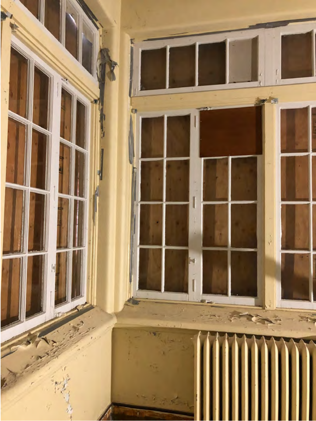
SUNROOM – wood casement windows in the sunrooms are in fair to poor condition
