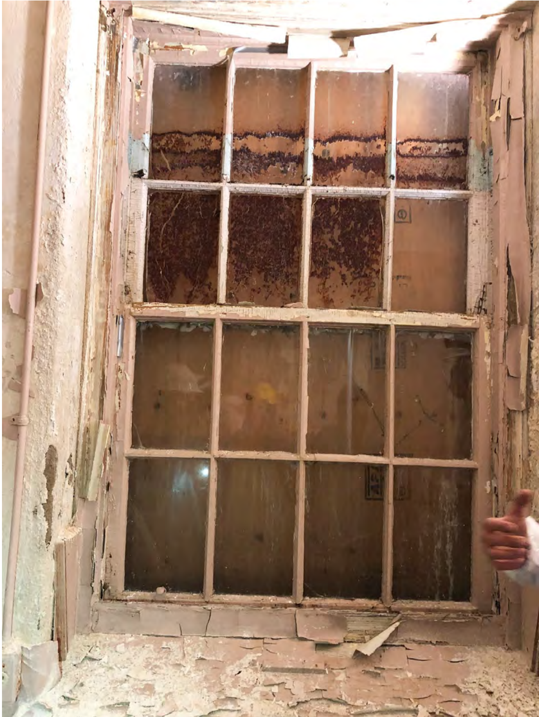
WINDOWS – 8 over 8 wood sash windows on the main elevation are in poor condition
