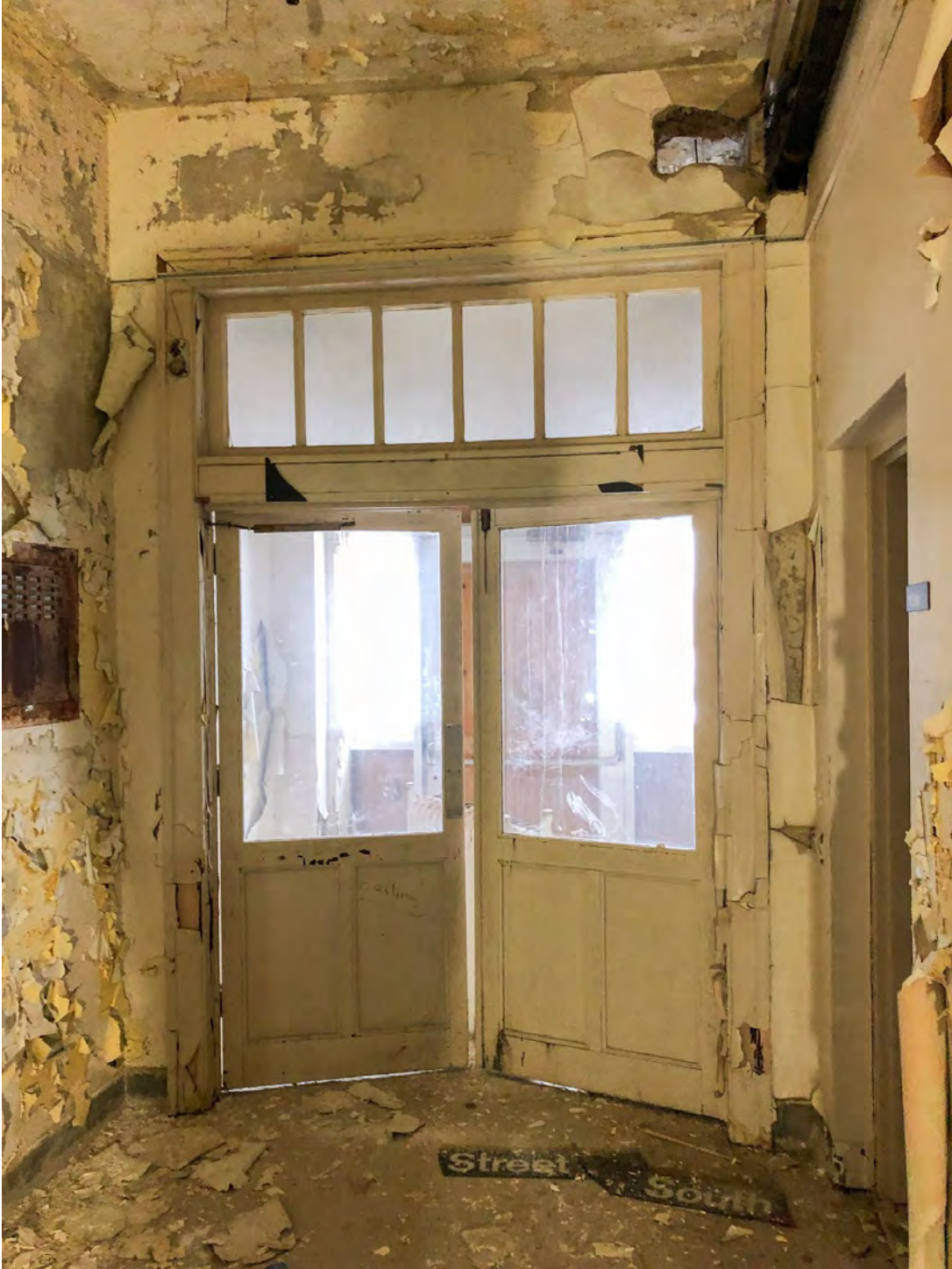
WOOD DOORS – wood doors with transom above are in fair to poor condition
