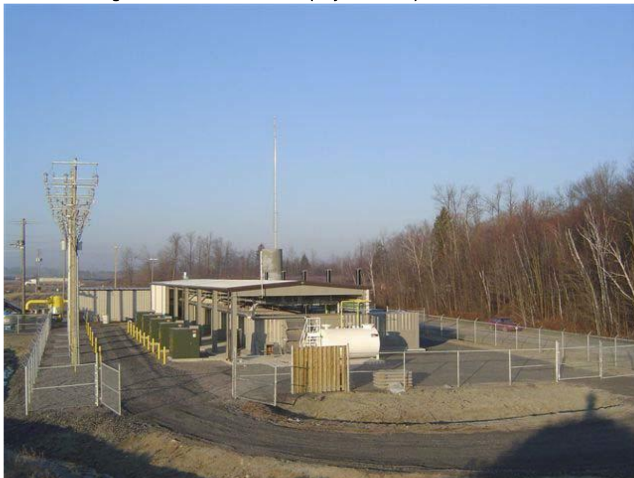
Figure 1 – Trail Road Landfill (City of Ottawa) 6 MW Power Plant
