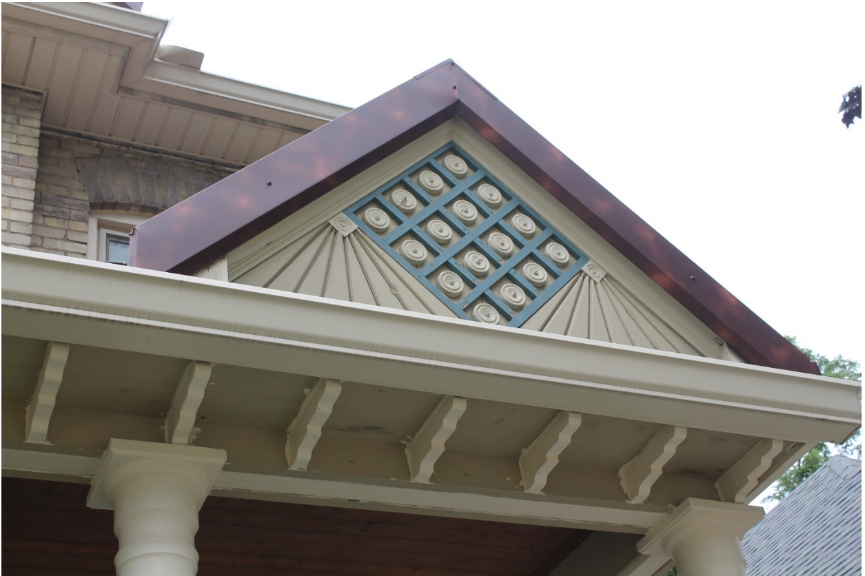
Image 8: Photograph showing the porch roof details, consistent with the detailing found in the gable of the dwelling.
