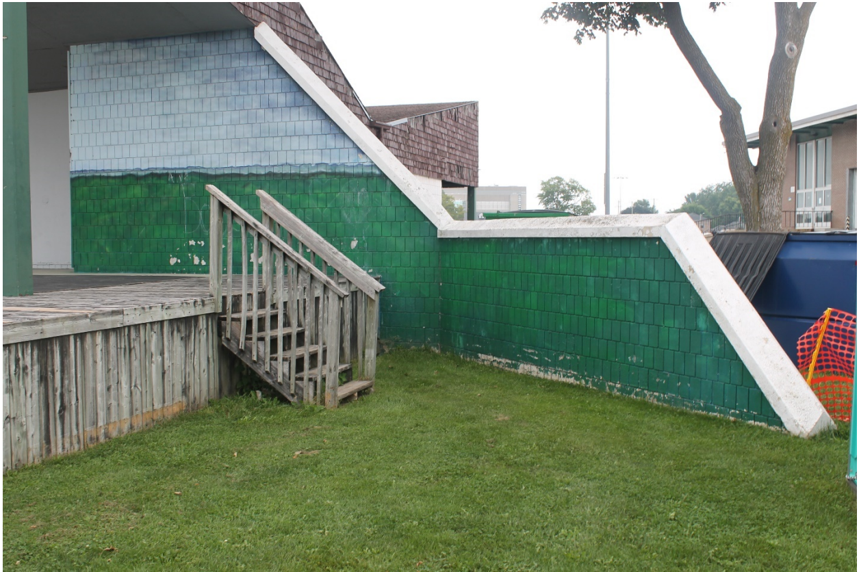
Image 4: Photograph showing the access to the south side of the Anne Eadie Park Stage, 2021.
