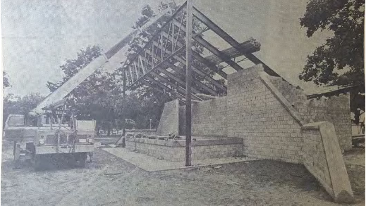
Image 1: Photograph showing the construction of the park stage at Queen's Park, as shown in the London Free Press, September 3, 1971.
