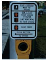
All AODA compliant push button
