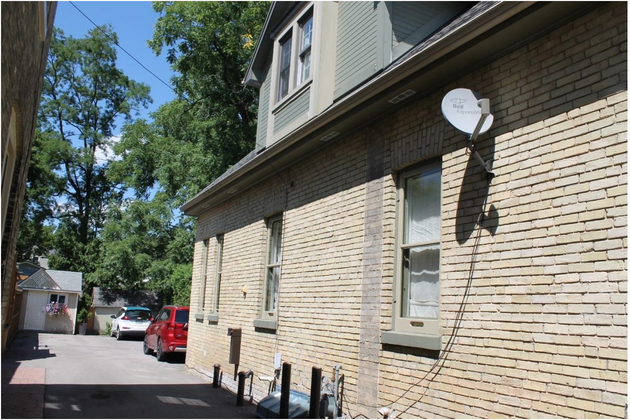
Image 9: Photograph showing the west facade of the dwelling and narrow right-of-way shared with the adjacent property at 44 Bruce Street.
