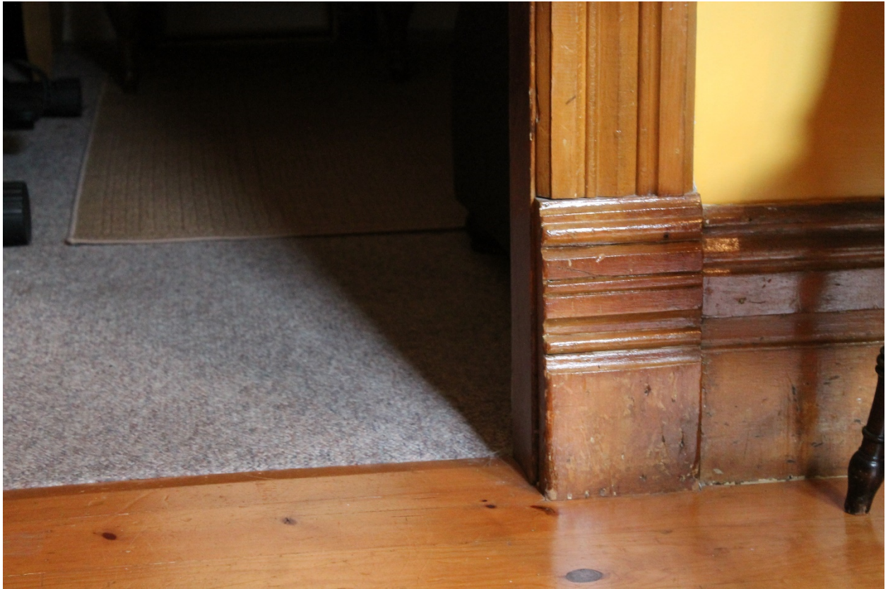
Image 17: Photograph showing detail of the baseboards on the interior of the dwelling.
