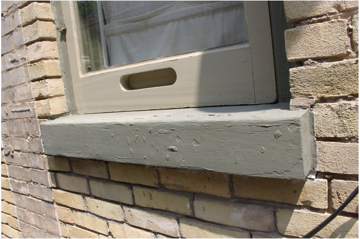
Image 11: Detail showing example of the wood sills found on the window openings for the dwelling.
