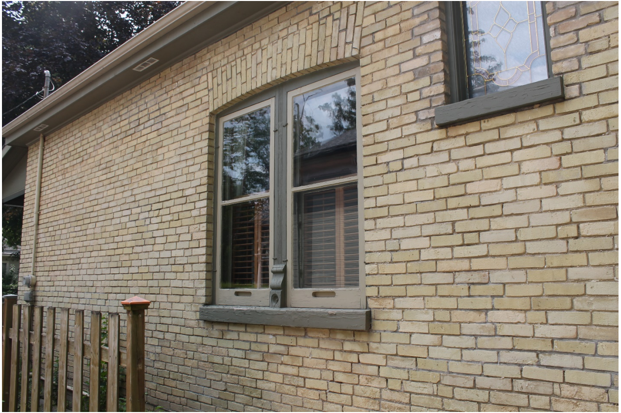
Image 15: Photograph showing the windows on the east facade including a pair of double-hung wood windows, a fixed window (later alteration), and details including voussoirs, carved mullion, and wood sills.
