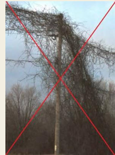
Guy-wire growth contacting electrical equipment & powerlines
