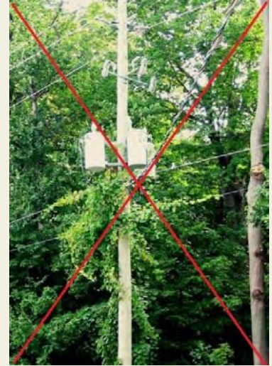
Pole growth contacting electrical equipment & powerlines
