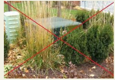
Obstruction around a transformer
