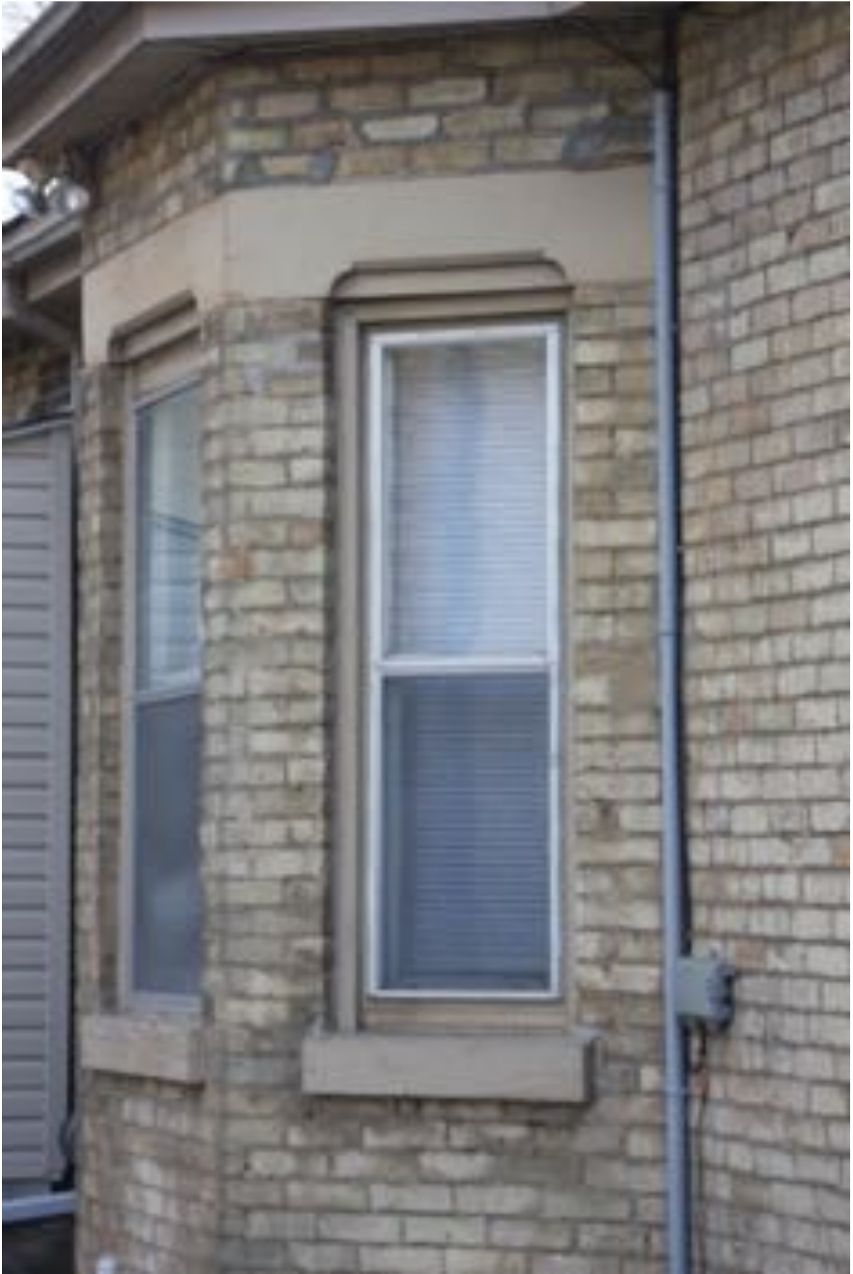
Close-up of bay window on the left side of 179 Ann Street, showing North Talbot lintel.
