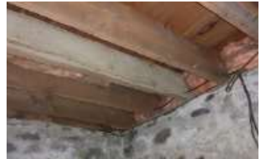
Image 8: Existing basement joists on rubble/fieldstone foundation. Photo Source: HIS, Stantec Consulting Ltd, April 2018.
