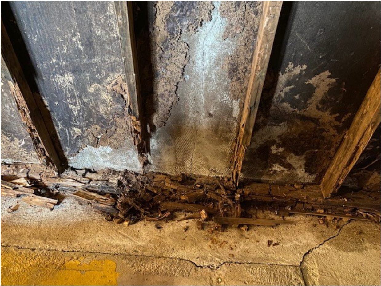
Image 5: Interior view of detached garage showing degradation of wood sill and wall studs (April 22, 2021)
