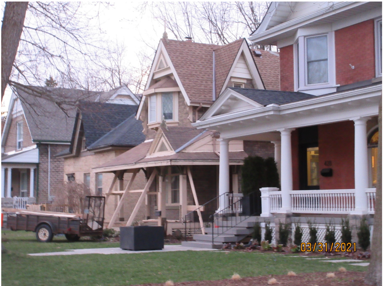
Image 3: Photograph, looking northwest towards the subject property, showing the alterations underway to the porch.
