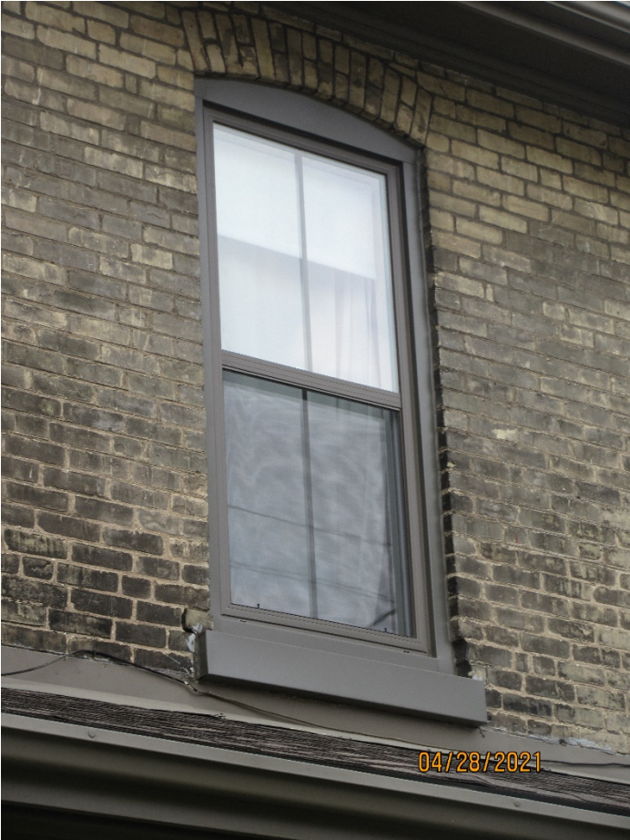
Image 10: Detail photograph of the replacement windows, showing the faux grille (muntin) of the replacement window. The faux grille is only between the glass panes and fails to accurately replicate any historic details.
