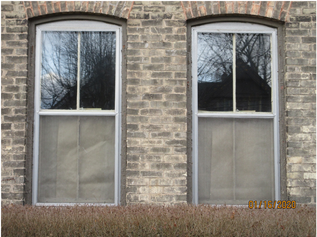
Image 5: Detail photograph of the exterior of the front windows (facing Askin Street) on the property at 40 Askin Street.
