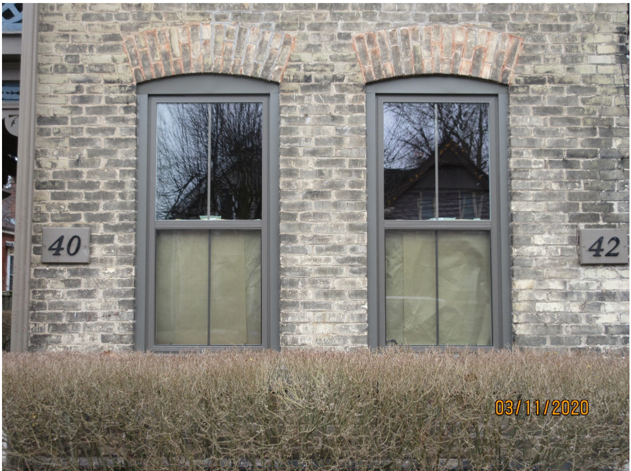
Image 8: Detail photograph of the replacement windows on the property at 40 Askin Street. Note that the insert windows do not fill the window opening and require capping, particularly as the replacement windows do not maintain the segmented arch shape of the window opening. The faux grille (muntin) lacks the authenticity of the former true divided light windows.
