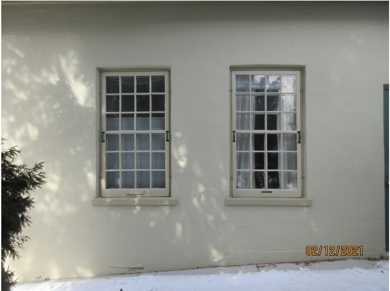
Image 23: Photograph showing the two twelve-over-twelve painted wood windows with storm windows and wooden sills on the south façade of Carfrae Cottage.
