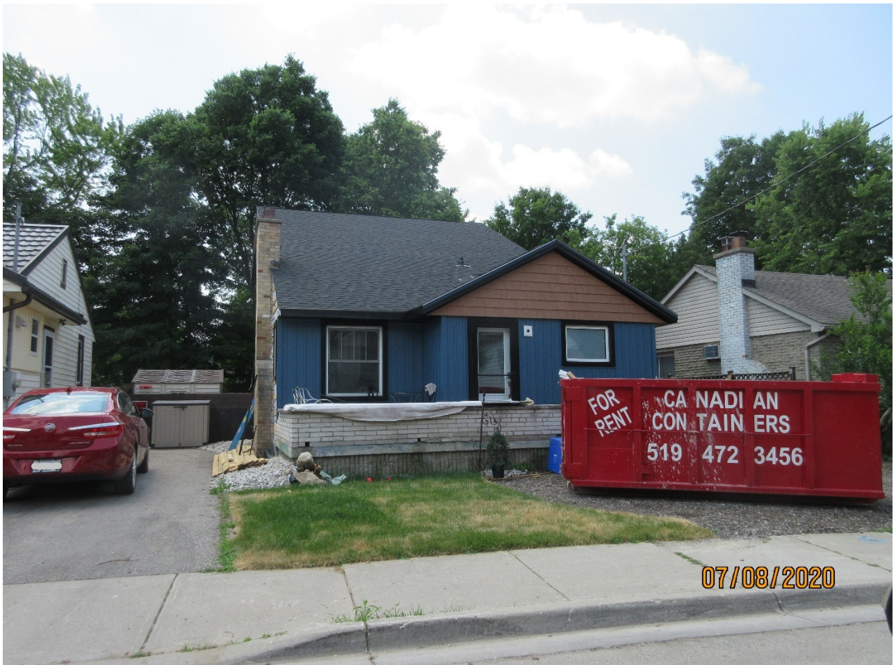
Image 4: Photograph of the subject property, on July 8, 2020, when non-compliance with the Heritage Alteration Permit was identified. Note the change in the exterior cladding, including gable, and the front door replacement. The shutters were also removed.
