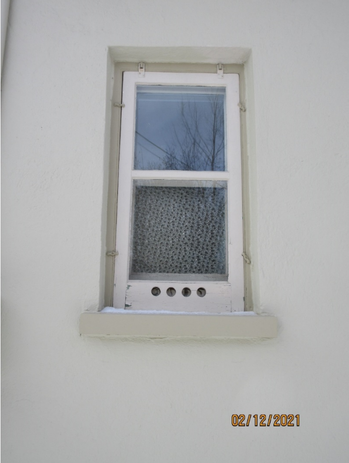
Image 32: Photograph of the bathroom window on the east façade with patterned glass in the lower lite and clear glass in the upper lite of the hung window with a storm window and wood sill.
