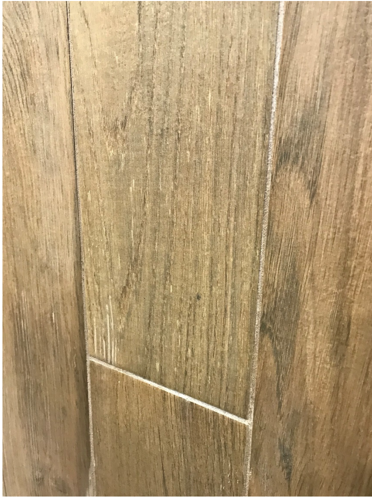
Image 7: Detail of faux wood grain porcelain tile installed on the storefront of the building at 181 Dundas Street.
