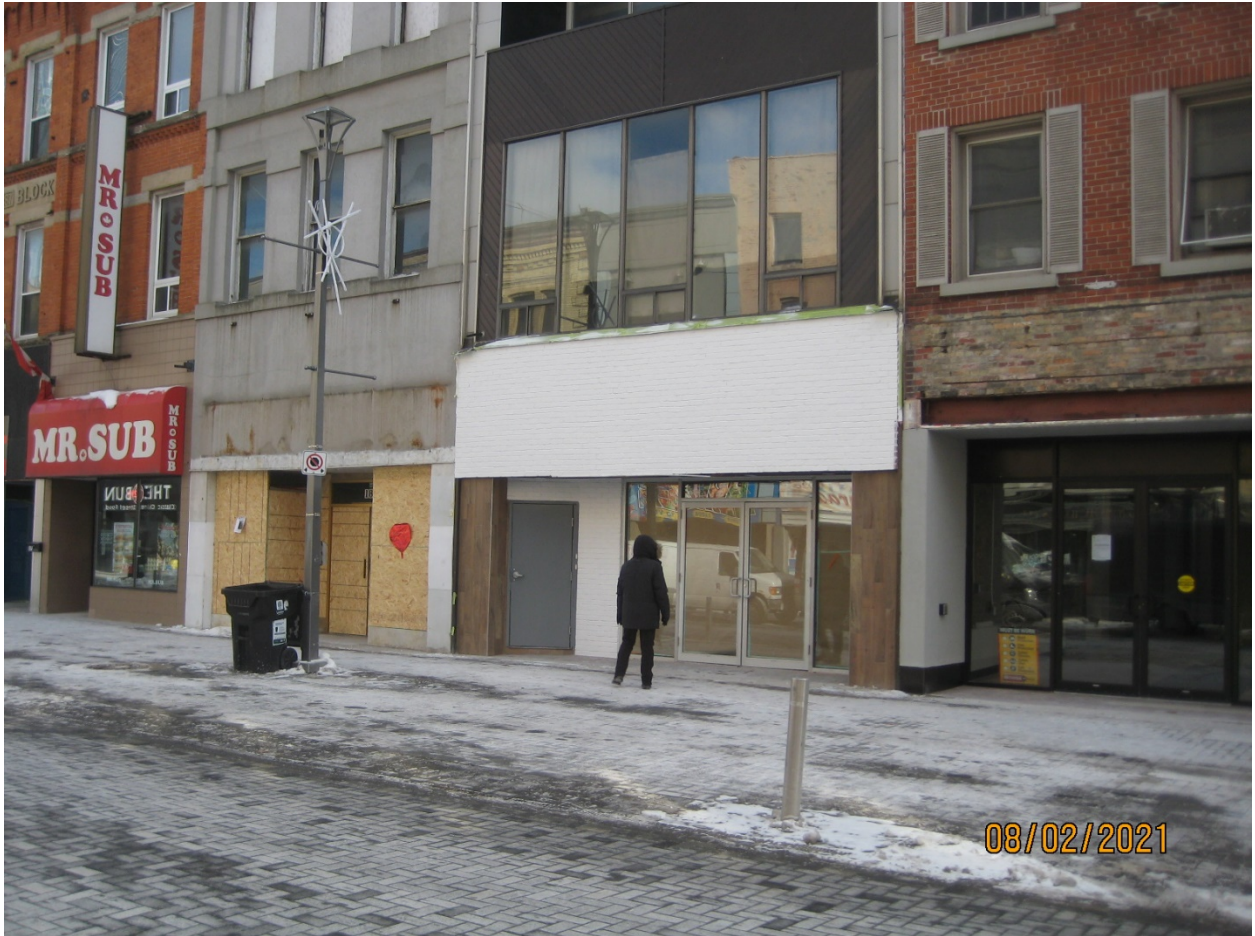
Image 5: Photograph of the property at 181 Dundas Street showing the unapproved alterations, including painted brick veneer and faux wood grain porcelain tile.
