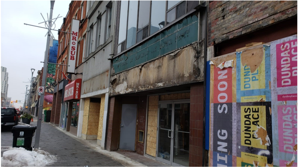
Image 3: Photograph of the building located at 181 Dundas Street following the removal of the backlit sign box, showing existing conditions in January 2021.
